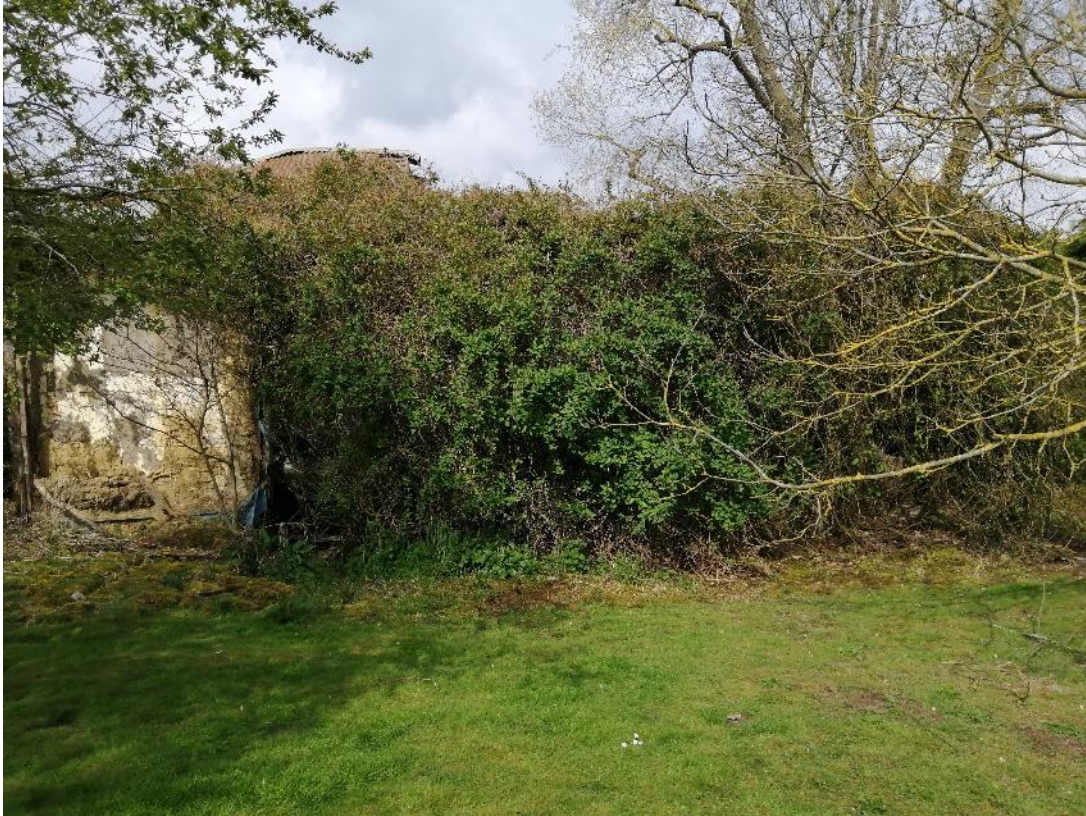
Photograph 7: East side of outbuildings overgrown with Russian vine
