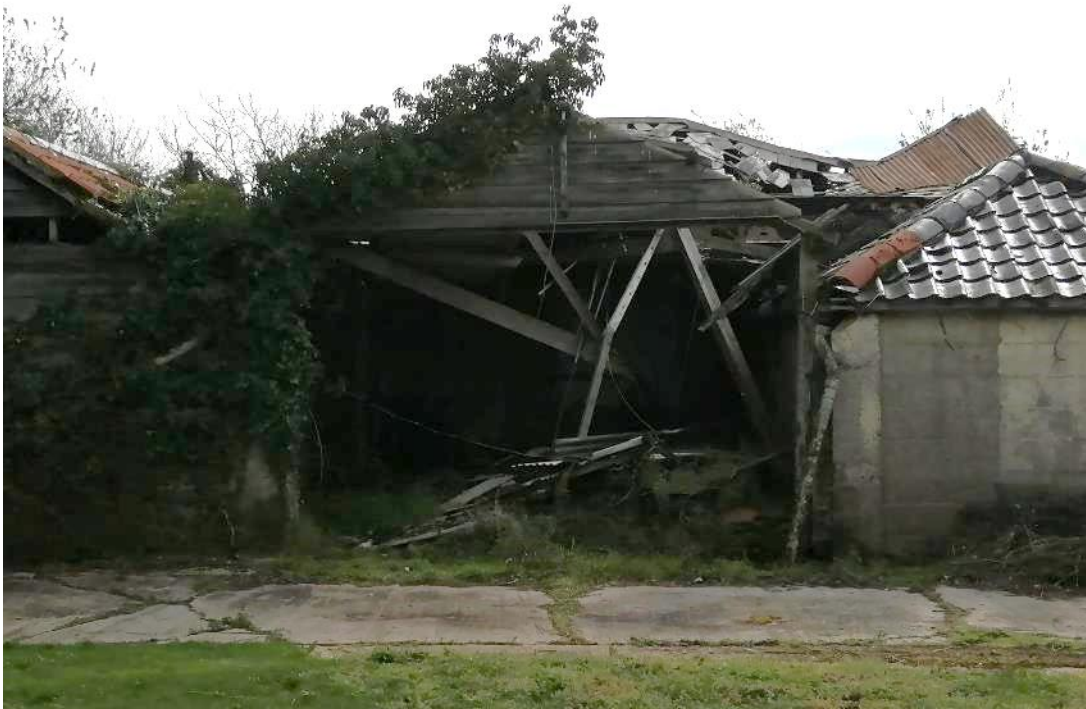
Photograph 6: Open-sided timber barn with collapsed roof (centre)
