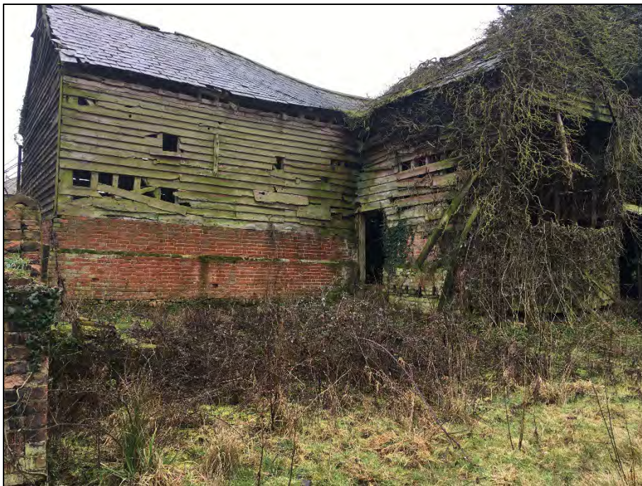
Photograph 24: The large barn adjacent to the western boundary, from the northern side. This barn had collapsed by December 2022, as shown in Photographs 39 and 40.
