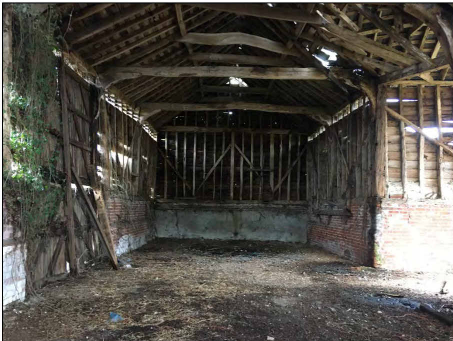
Photograph 26: Inside the large farm building. This barn had collapsed by December 2022, as shown in Photographs 39 and 40.
