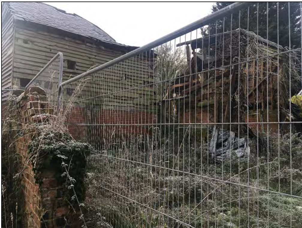
Photograph 39: The collapsed barn on the western boundary. The barn standing in March 201 is shown in Photographs 24 – 26 and 30.
