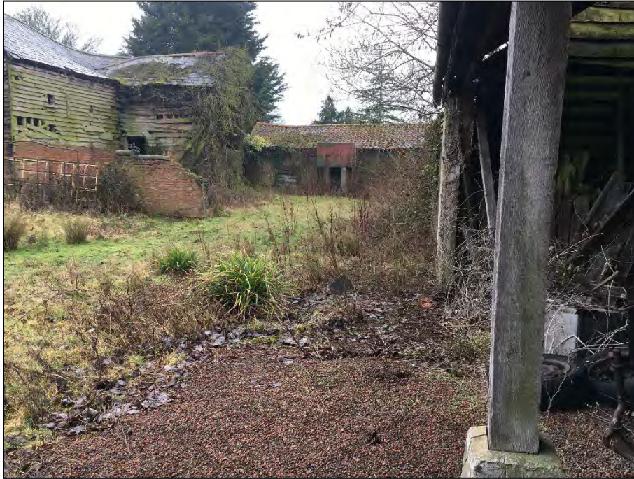
Photograph 15: The north-western sector of the site, also showing an above ground fuel storage tank adjacent to a building.
