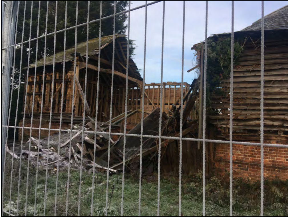
Photograph 40: The collapsed barn on the western boundary. The barn standing in March 2011 is shown in Photographs 24 – 26 and 30.
