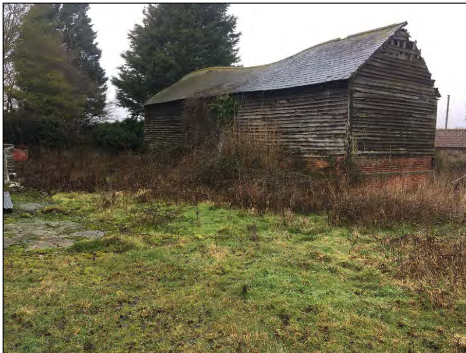
Photograph 30: The south side of the large farm building adjacent to the western site boundary. This barn had collapsed by December 2022, as shown in Photographs 39 and 40.
