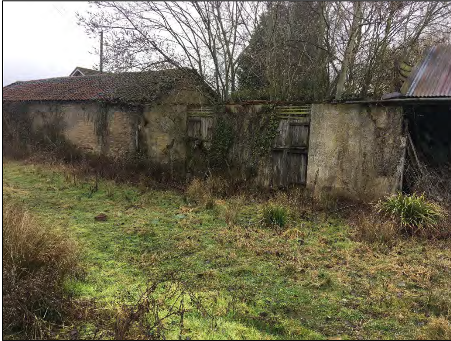
Photograph 21: The row of buildings in the western sector, alongside the northern site boundary. The building in the centre of the photograph was derelict with the roof and the northern wall missing.
