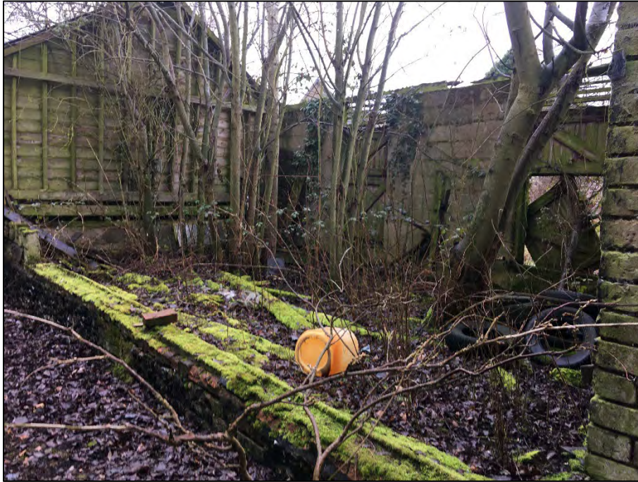
Photograph 33: The derelict building within the row of buildings on the northern site boundary.
