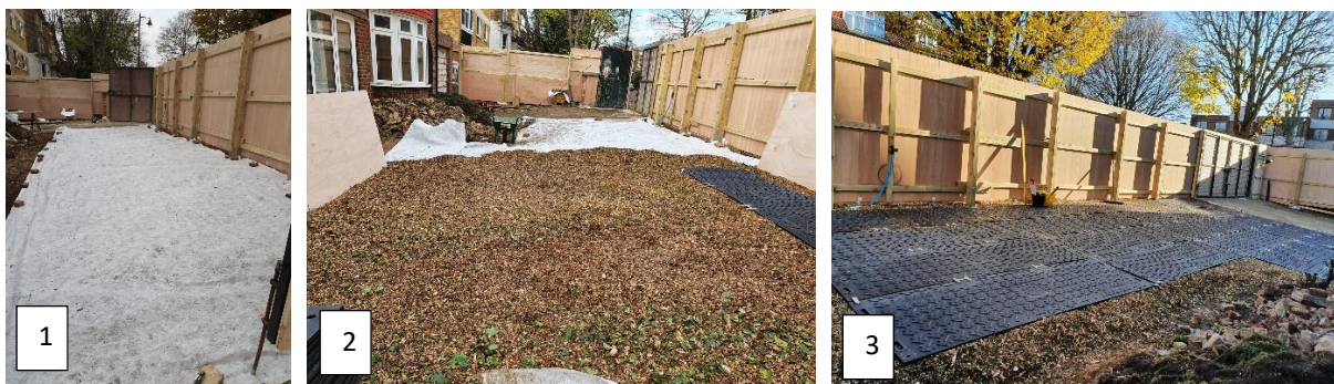
Images above from a site managed by Usherwood Arboriculture and showing the three stages of ground protection installation.
