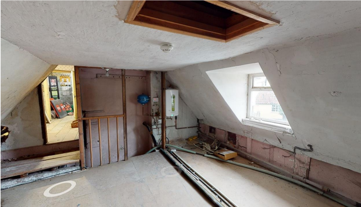
Interior view of first floor void area to be incorporated in to vaulted ceiling above sales area extension, looking towards the head of the redundant stair
