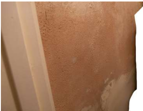
Fig 3.5 Damp patch in Larder of No 4 where studded cavity membrane to be installed to damp wall. Plaster to be removed first
