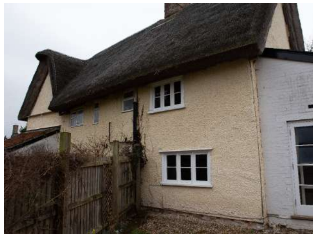
Fig 1.11 No 6 Church Way from NW. No 4 beyond fence which is to be removed. Note gaps to render at corners that will be repaired like for like.
