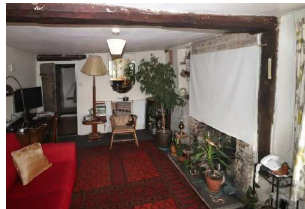
Fig 3.7 No 2 Church Way LivingRoomshowing fireplace at right to receive insulated soffit board and vent. Photo - Hoggett HIA>
