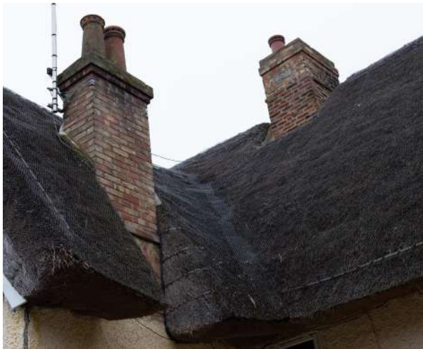
Fig 4.1. 19th C chimney stack with defective cement flashing to be replaced with lead
