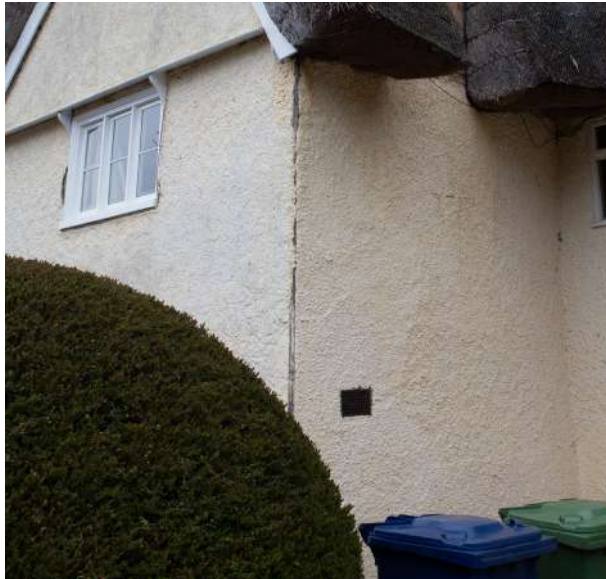
Fig 4.0. Gaps in approx 1930s roughcast cement external finish that require repair
