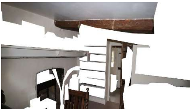
Fig 3.9. First floor beam to No 4 Living area fixed into central chimney structure.
