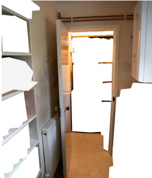
Fig 3.4 Location of Proposed Ground Floor Doorway (straight ahead) from No. 4 Kitchen showing modern doorway/partition and shelves to Larder to be removed.
