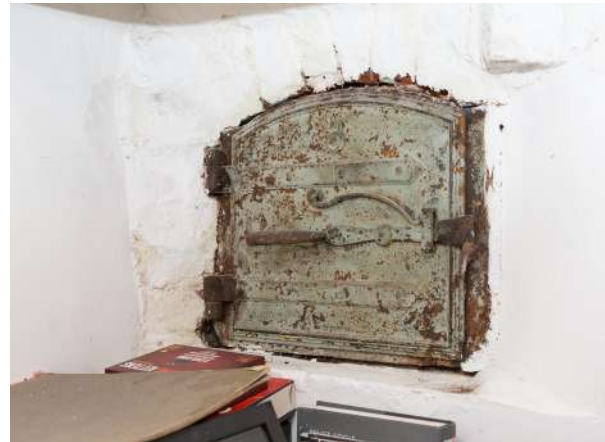
Fig 3.2 Metal door to bread oven in No 6 Living Room which is deteriorating due to damp surrounding brickwork to unventilated oven.
