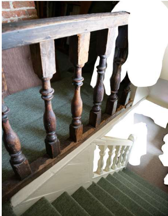
Fig 3.8. Historic staircase to No 4 dated to early 18th C. Of a level of elaboration that is likely from before the property subdivision and is designed to fit with the brickwork central chimney (background).
