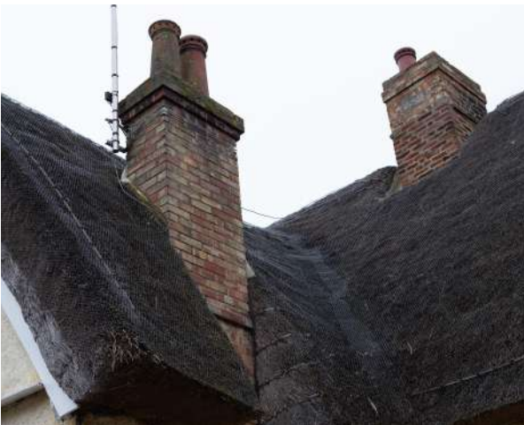
Fig 4.2. Cracked cement flashing and unsuitable cement pointing to chimneys
