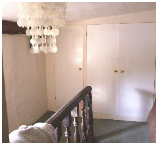
Fig 3.2 Landing of No 4 showing modern cupds to be removed and wall beyond to receive new open doorway to No 6.
