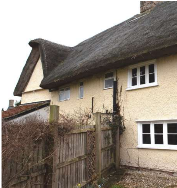
Fig 5.1. Existing modern boundary fence between rear gardens of No 4&6 to be removed.
