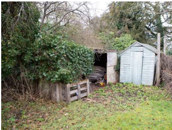
Fig 5.2. Existing sheds to garden of No 4 in poor condition and to be removed and replaced with single shed in garden to No 6.
