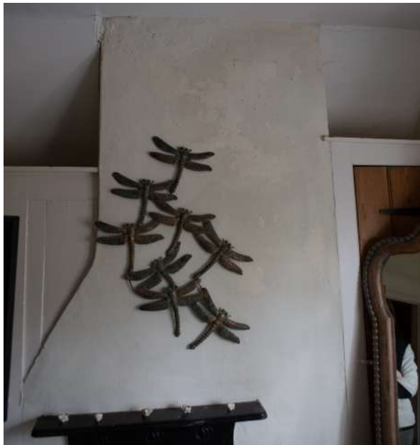
Fig 4.1. Area of damp to chimney breast within Bedroom 2 in No 6.
