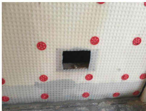
A disused chimney breast being lined with RUK Slimline before plastering. A grille was fitted to ventilate the disused flue.
