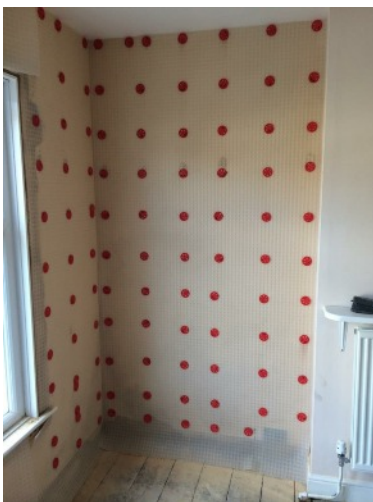
An alcove with slight penetrating damp lined with RUK Slimline then insulated plasterboard & skim
