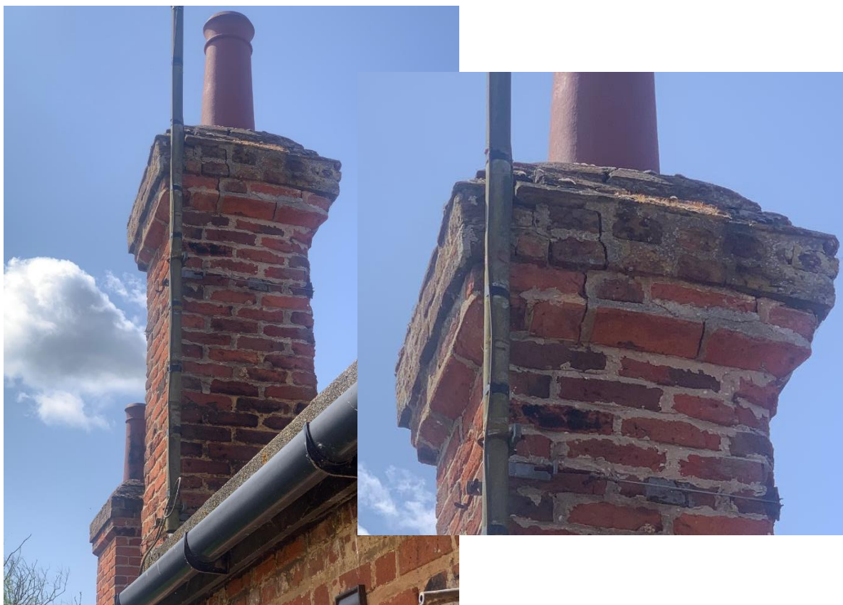
Figure 9: Damage to chimney on Western elevation
