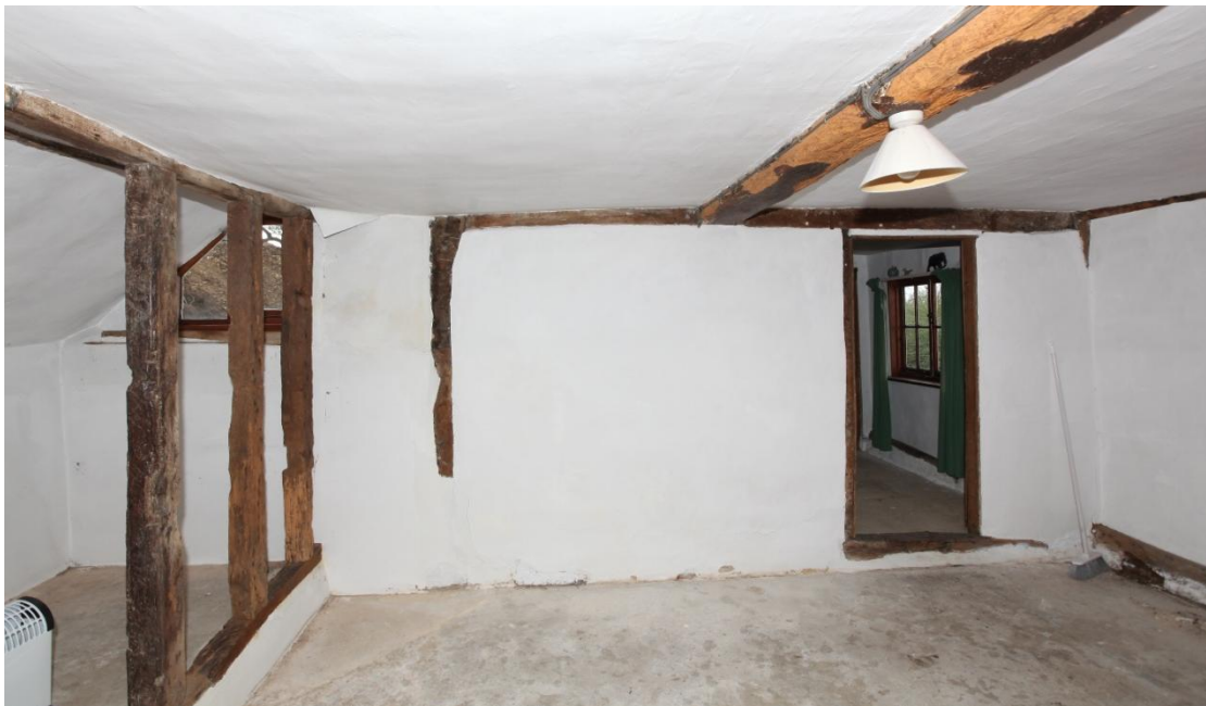
Illus. 16. The south-western wall of the dining room with the door to the 'lounge' on the right. The isolated jowled post to the left marks the position of the original back wall and the present studs lie within the lean-to. The axial joist is central to the present room, suggesting the ceiling may have been rebuilt when this room was widened.
