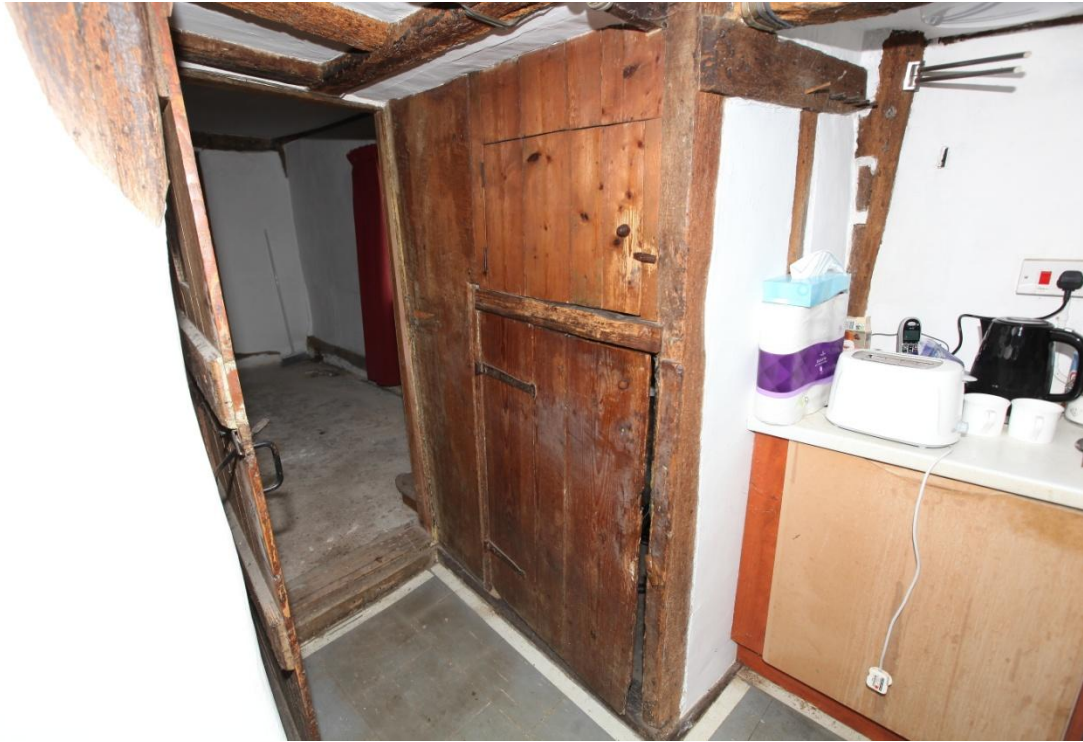
Illus. 7. The mid-19 th century pine boarding to the stair in the corner of the kitchen which is respected by a trap in the ceiling joists. These timbers date from the 17 th century or earlier but are not pegged and have been re-used.
