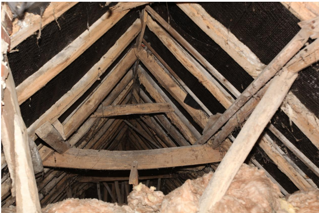
Illus. 26. The roof structure seen from the axial chimney to the north-east. The rafters consist of a variety of re-used timbers with pegged collars and clasped-purlins. The presence of a ridge-board indicates a degree of alteration in the mid-19 th century.
