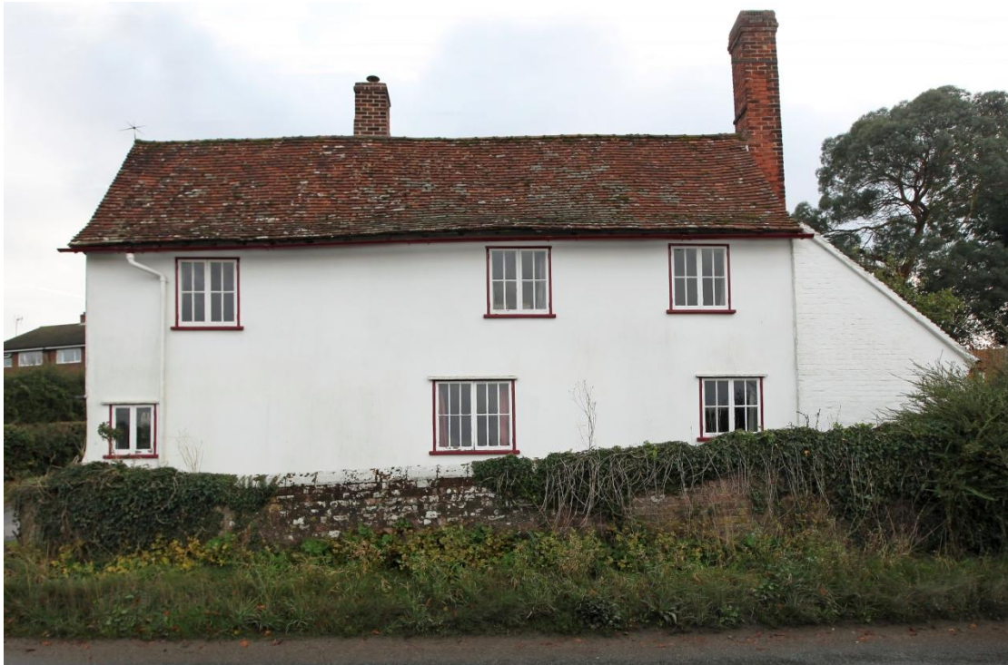
Illus. 1. The north-western facade with the substantial mid-19 th century brick lean-to on the right and the uniform late-20 th century casement windows with narrow lights that differ from those shown in the 1960s photographs (figures 8-9). The present windows were inserted as part of an extensive renovation in or about the 1980s, with only the ground-floor window to the right replicating its predecessor of 1961.
