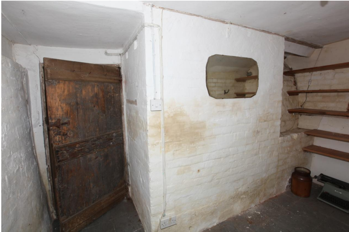
Illus. 19. The back of the 'lounge' chimney from the mid-19 th century lean-to against the south-western gable. A straight vertical joint divides the chimney from the brickwork to its right, suggesting the lean-to may slightly post-date the chimney. The curious curved section above may survive from a former bread oven in the position of the present 'lounge' cupboard but there is no other evidence to support this.
