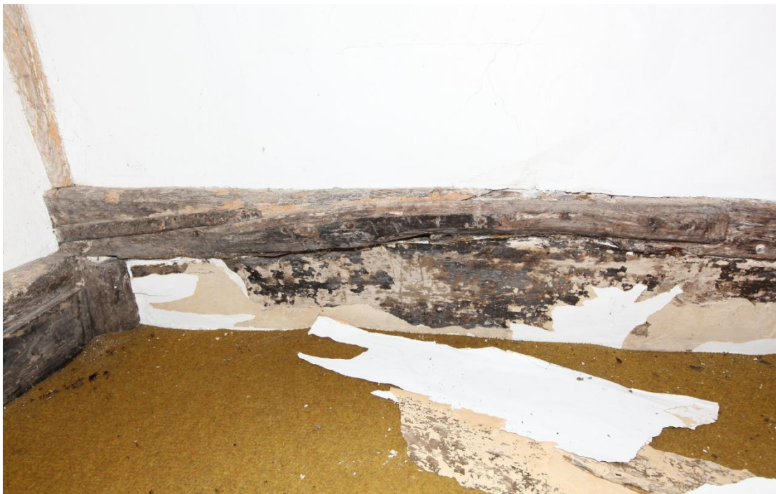
Illus. 22. A detail of the low north-eastern tie-beam in illustration 21 (bedroom 1) showing a diagonally splayed joint secured by a nailed length of characterful roughwood. A tie-beam should not contain a joint of any kind and the presence of this feature indicates a significant degree of alteration or reconstruction.
