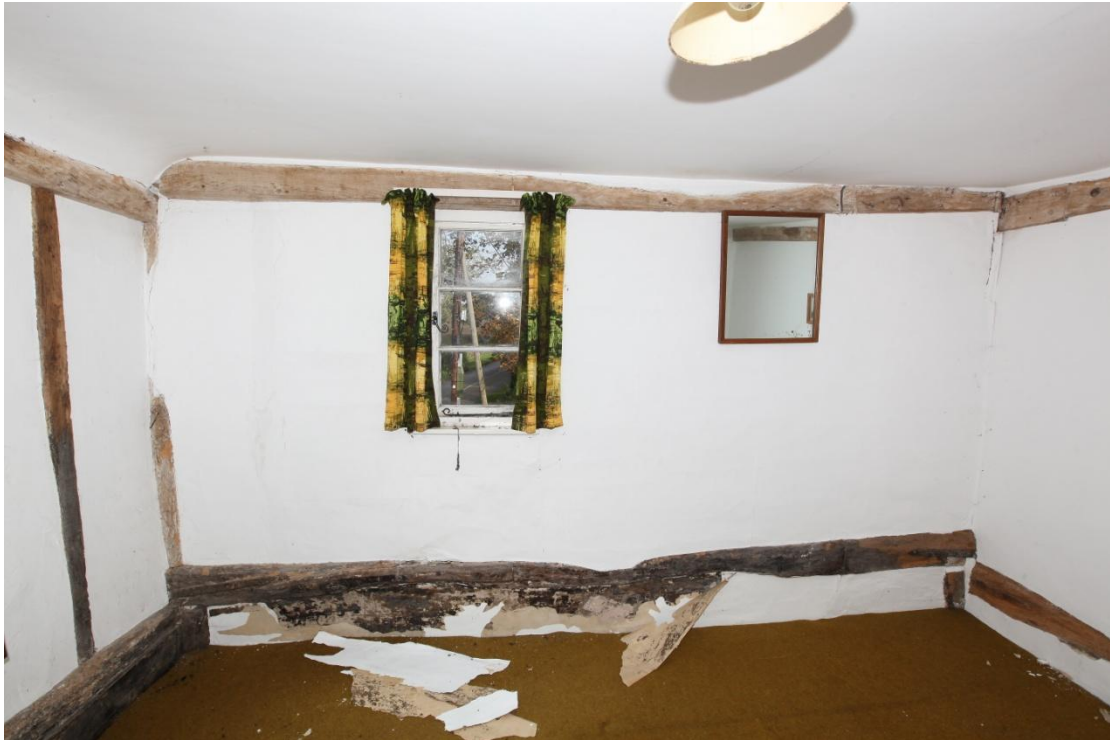
Illus. 21. The interior of the north-eastern gable, facing Church Lane. The low tie-beam rests on jowled corner posts with corresponding roof-plates just above the floor and survives from an earlier single-storied building to which the present upper storey was added in the 18 th century. A number of anomalies including a joint in the tie-beam (illus. 22) indicate that this earlier timber frame was either extensively rebuilt as part of the process or consisted of re-used material from the outset.
