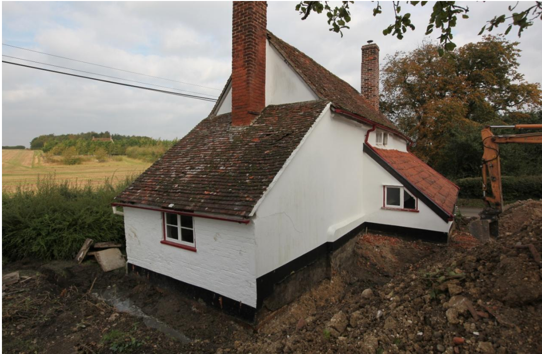
Illus. 5. The brick lean-to against the south-western gable was added as part of the mid-19 th century refurbishment and the historic maps suggest the pantiled lean-to once continued to its right-hand corner. The late-20 th century window in the latter's present gable is consistent with a recent truncation or reconstruction, as is the absence of a rear window in the service bay (i.e. the 'lounge' in figure 10).
