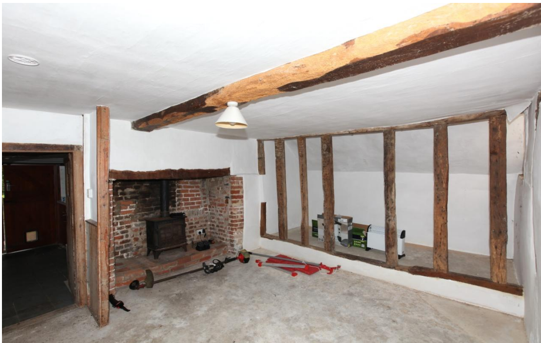
Illus. 12. The hall ('dining room') from its western corner showing the rear lean-to on the right and the door to the kitchen on the left. The original back wall adjoined the fireplace but has been moved into the lean-to by approximately 2 feet.
