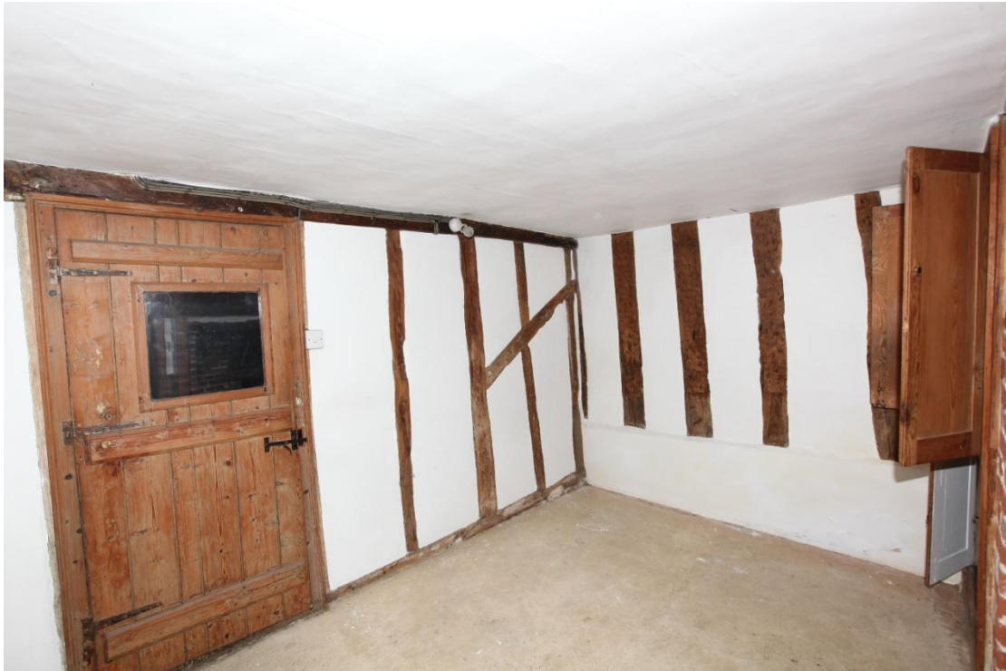
Illus. 17. The narrow service room ('lounge'), showing the chimney against its south-western gable on the right and the door to the hall ('dining room') on the left. The substantial studs in the back wall date from the 17 th century or earlier but unlike their counterparts in the hall do not correspond with the pegged mortices in the exposed roof-plate on the upper storey. The narrow studs and diagonal brace of the internal partition are typical of the 18 th century but the mid-rail above is in two sections linked by a splayed scarf joint in a manner that suggests the timbers have been re-used.
