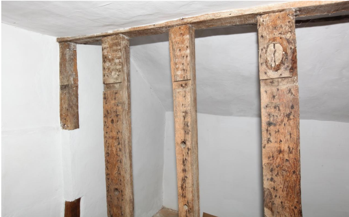
Illus. 13. A detail of the studs in the back wall of the ‘dining room’ (illus 13). In addition to the scars of lath-and-plaster these 17 th century timbers contain grooves that were normally cut into the external surfaces of contemporary walls to secure external wattle-and-daub, indicating they have been re-used. Their upper ends are now nailed and tenoned to a rail which lies beneath the roof of the lean-to, but the attachments are not modern and they may have occupied their present positions since the 19 th century.
