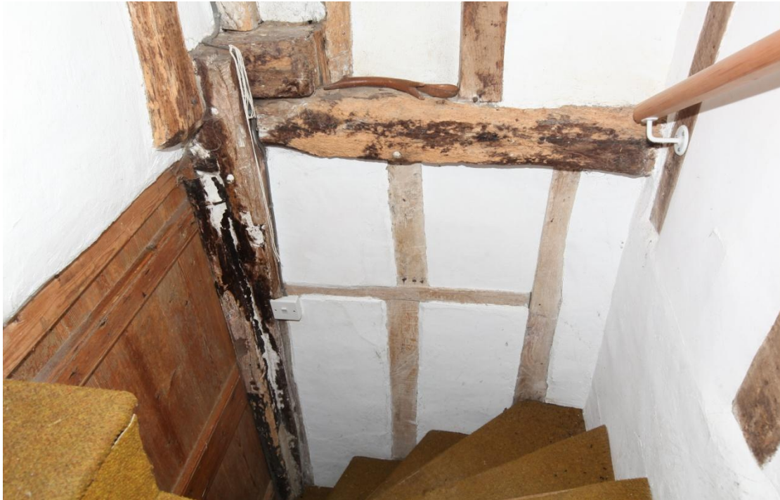
Illus. 15. The front wall adjoining the stair with clear evidence of a blocked lobby entrance door: the horizontal lintel corresponds with a rebate in the jowled post on the left. The post contains mortices for a mid-rail and wall brace similar to those in the corner of the kitchen which is hidden to the right (illus. 8), and these two posts appear to have formed a narrow bay for the chimney in a manner often seen elsewhere. The crude manner in which the roof-plates overlap suggests either that one was added as an extension to the other or they were re-used in the original single-storied structure. The ostensibly in situ narrow wall studs are typical of the 18 th century.
