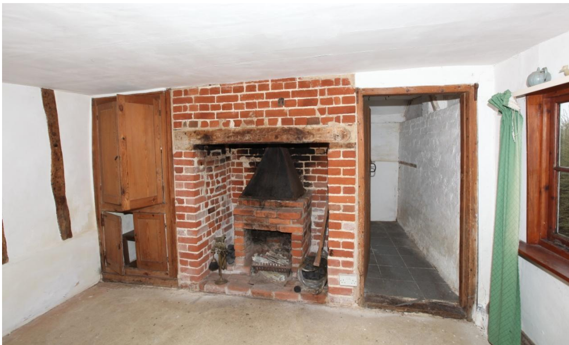
Illus. 18. The fireplace against the south-western 'lounge' gable with the lean-to beyond. The uniform nature of its soft red bricks indicates this fireplace post-dates that in the 'dining room' and was added when the house was divided in the early-19 th century. The pine cupboard doors are likely to survive from the mid-19 th century remodelling.
