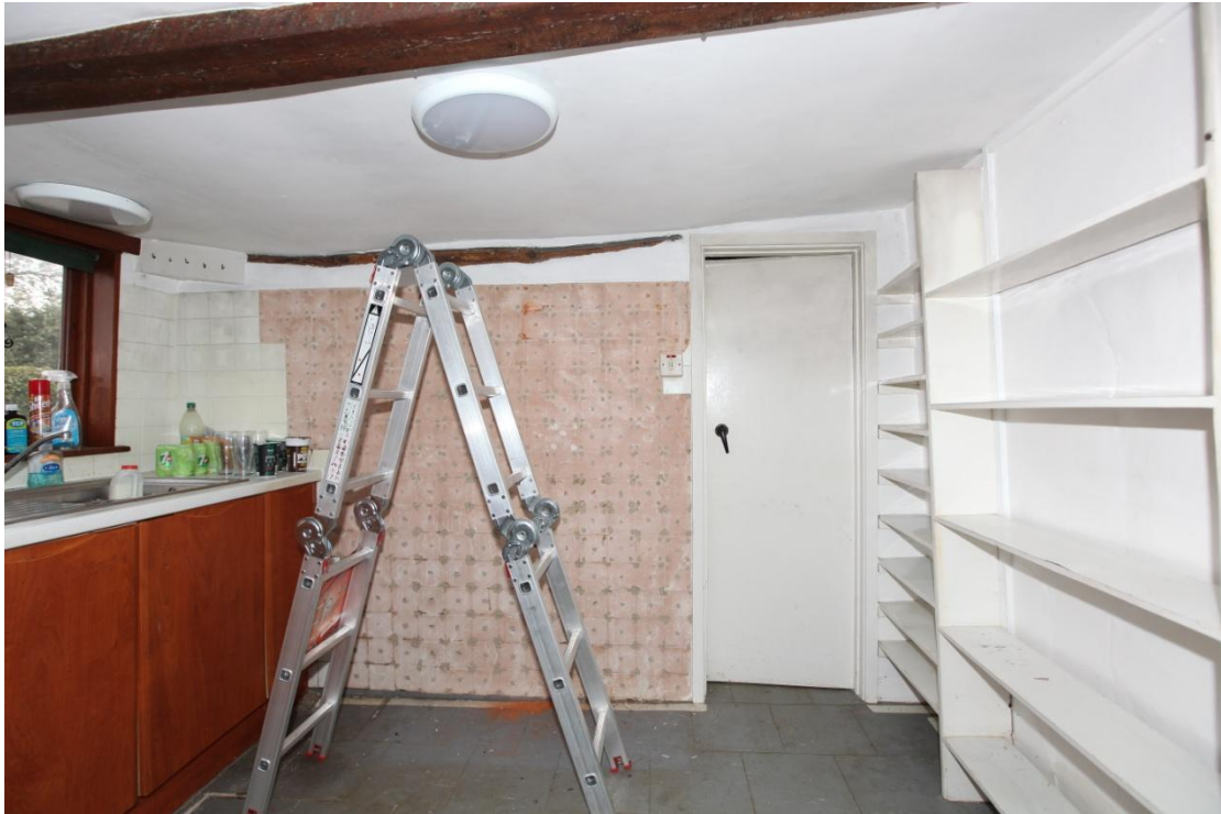
Illus. 9. The back wall of the kitchen with the entrance to the bathroom in the lean-to extension on the right. The exposed horizontal rail supporting the ceiling joists consists of 19 th century pine but the exact nature of the wall fabric beneath is unclear (see illustrations 10 and 11).
