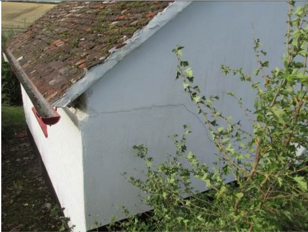
Photograph 07 – End lean-to settlement cracks to south corner
