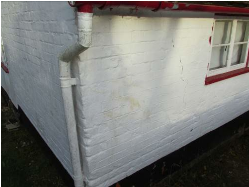
Photograph 08 – End lean-to settlement cracks to west corner
