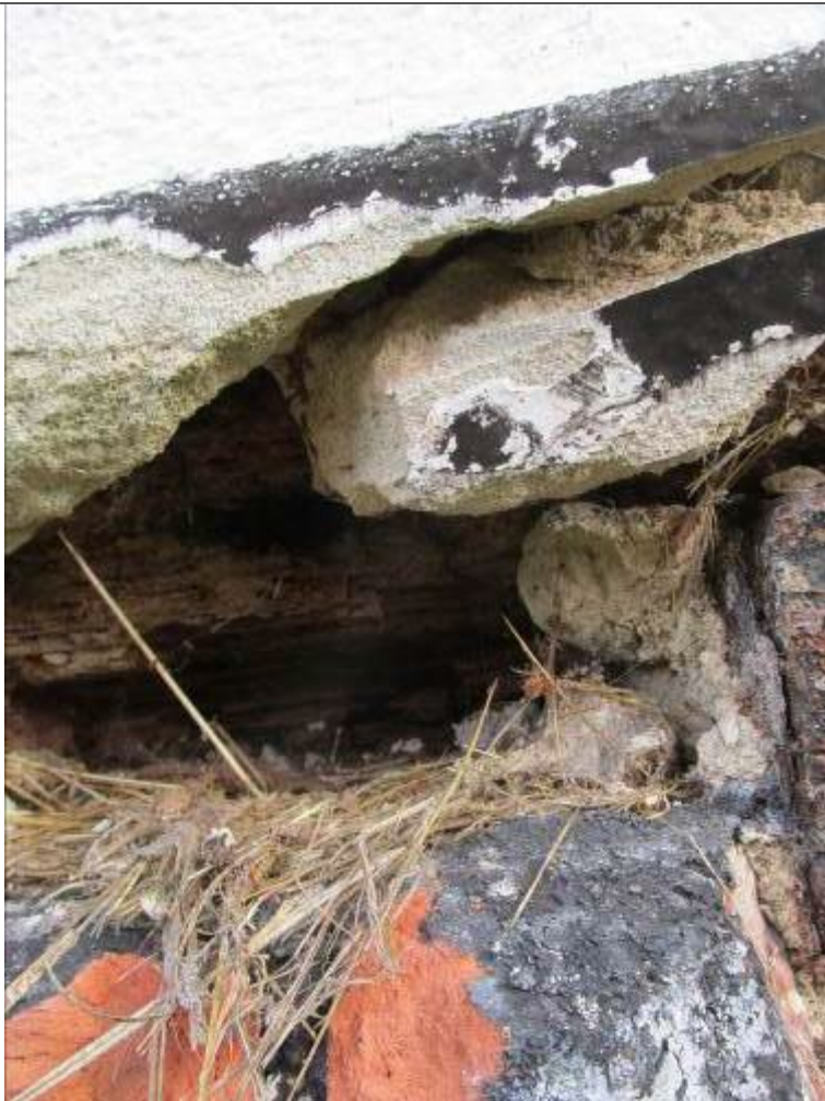
Photograph 06 – Trail investigation reveals poor condition of soleplate, expected to be typical, but will be uncovered as cement render is removed
