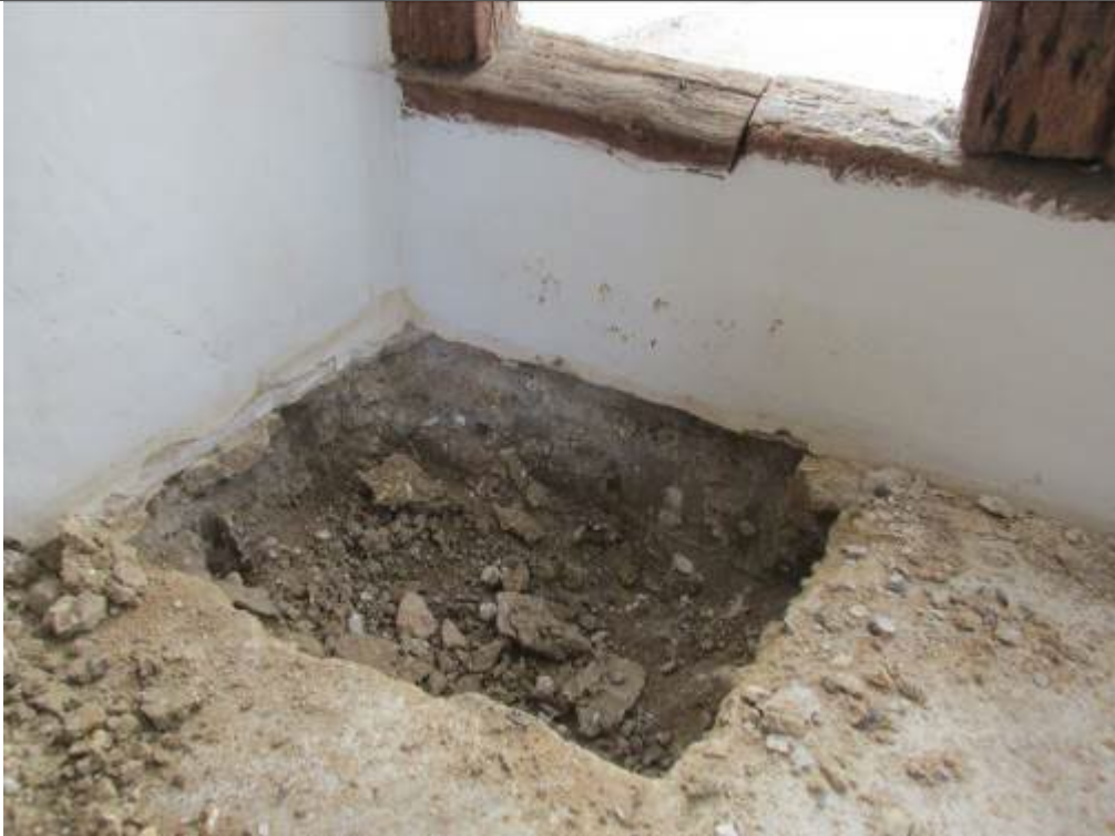
Photograph 05 – Trial pit typical against main chimney stack and rear lean-to internal, wall base at floor level directly onto earth
