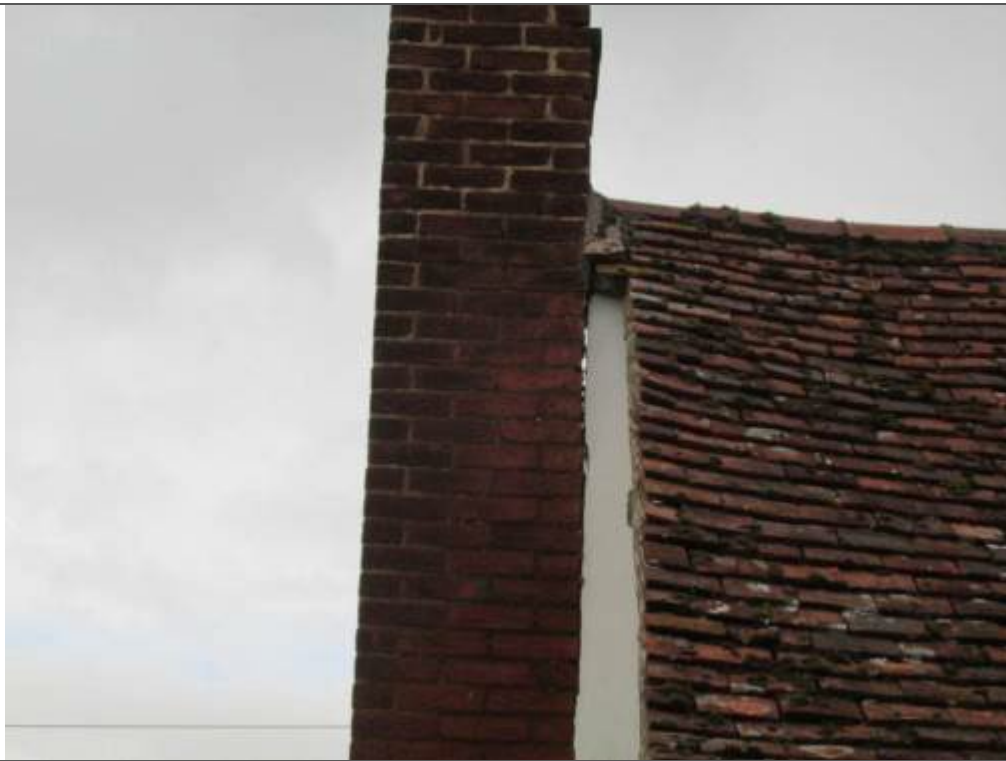
Photograph 16 – Slight separation between gable chimney stack and timber frame, where protective cover flashing is proposed to verge of tiles
