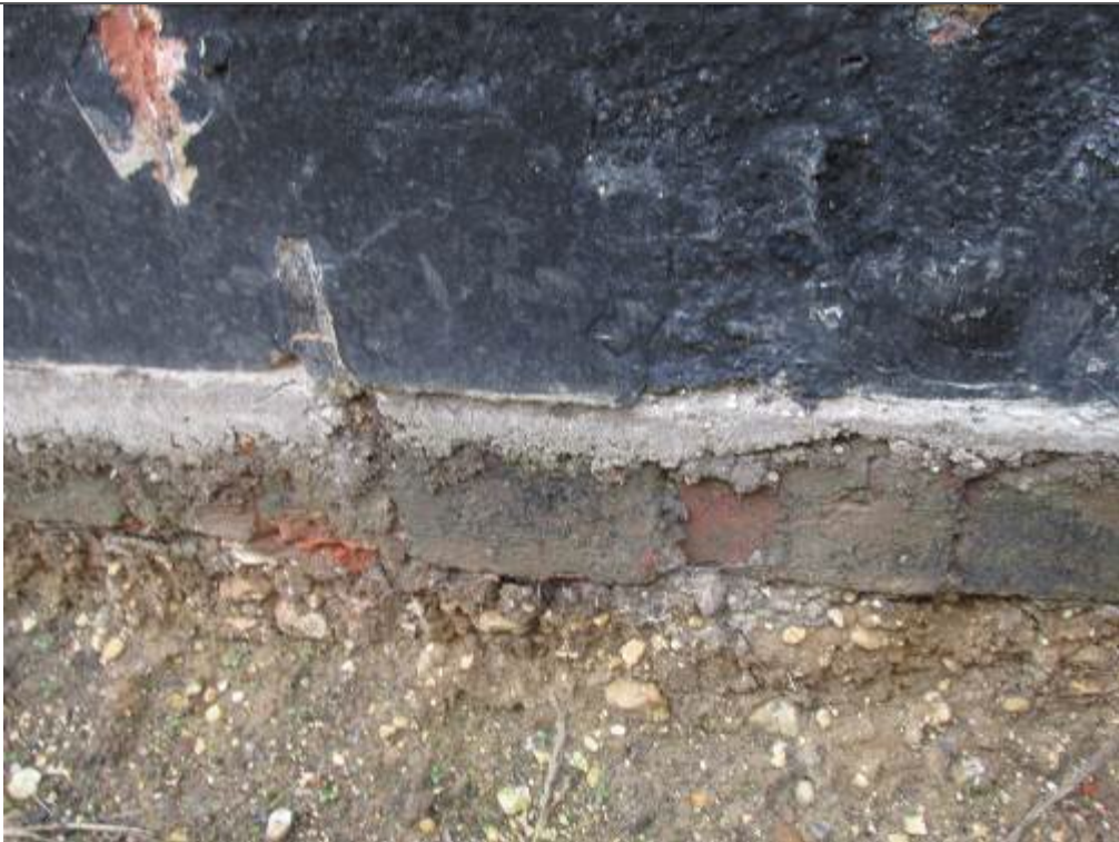
Photograph 04 – Trial pit typical, end lean-to with single course of brick below ground level, directly onto earth
