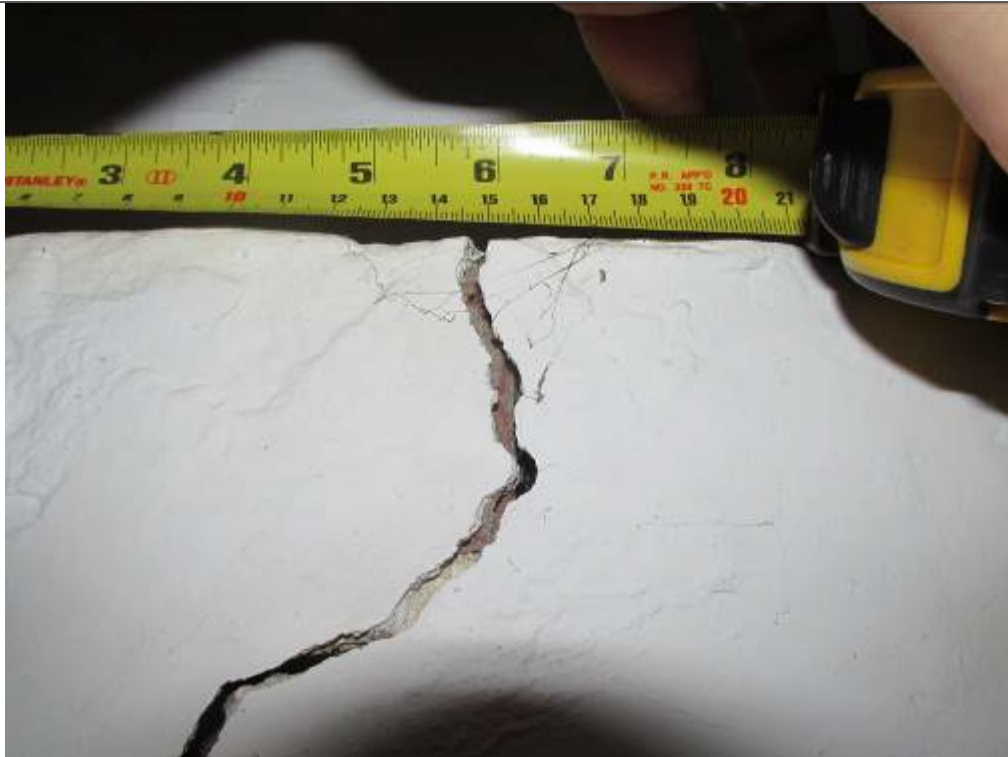
Photograph 13 – End lean-to settlement cracks measured internally
