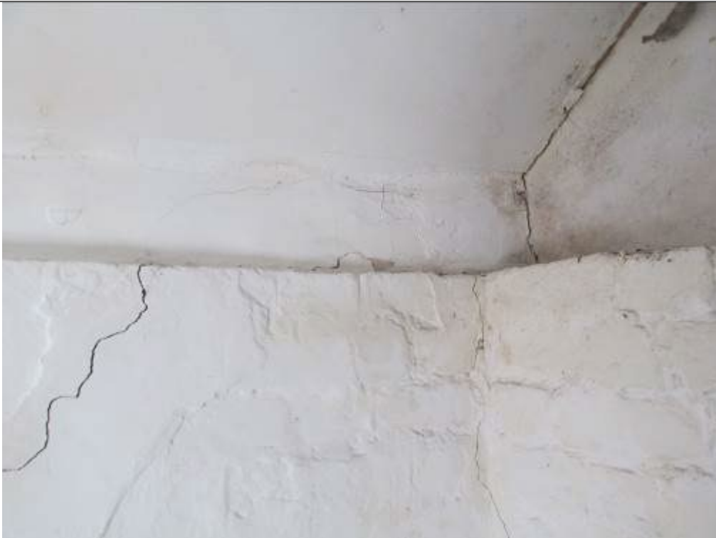
Photograph 12 – End lean-to settlement cracks to west corner (internal), typical, similar seen to south corner
