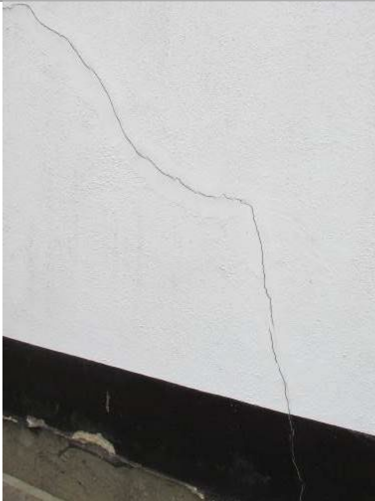
Photograph 15 – Rear lean-to differential crack adjacent to bathroom
