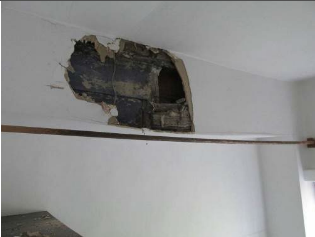
Photograph 18 – Wall frame over kitchen partition to be strengthened to allow modern fletton brickwork to be removed
