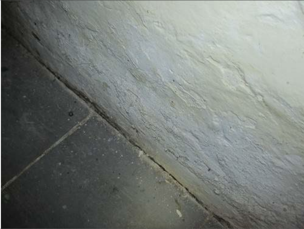
Photograph 11 – End lean-to separation of north wall of floor due to rotation
