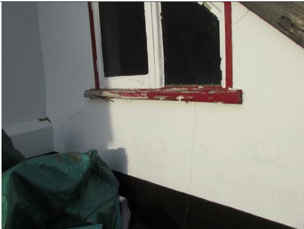
Photograph 14 – Rear lean-to settlement cracks
