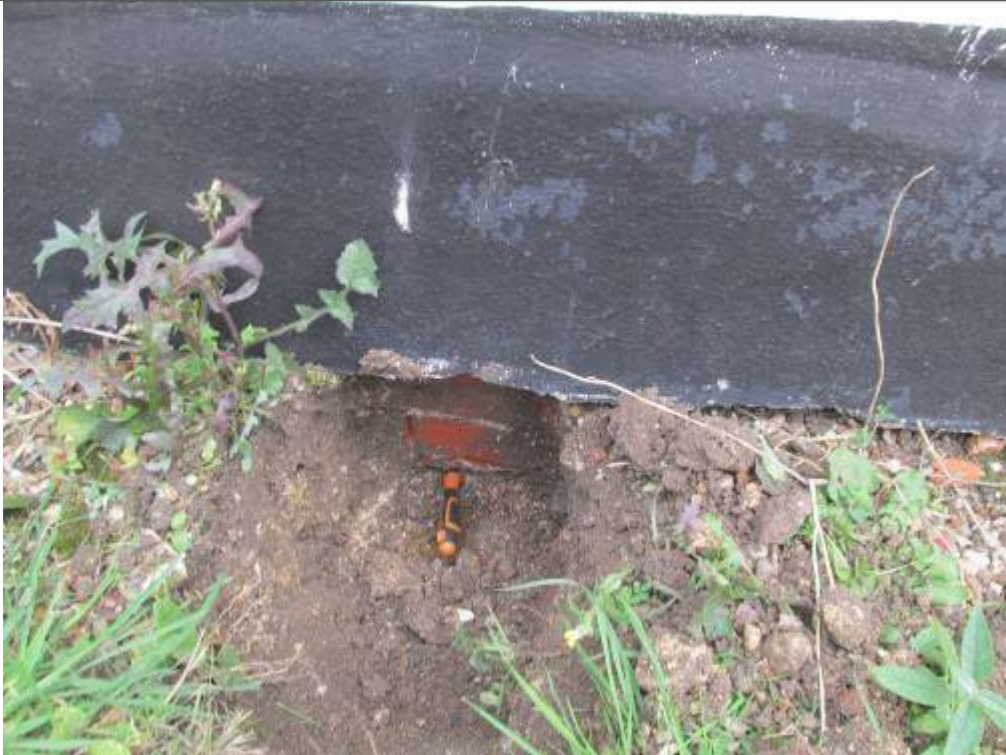
Photograph 03 – Trial pit typical, inspect walls/foundation shallow depth to plinth to timber frame walls (formation level identified at screw driver position)
