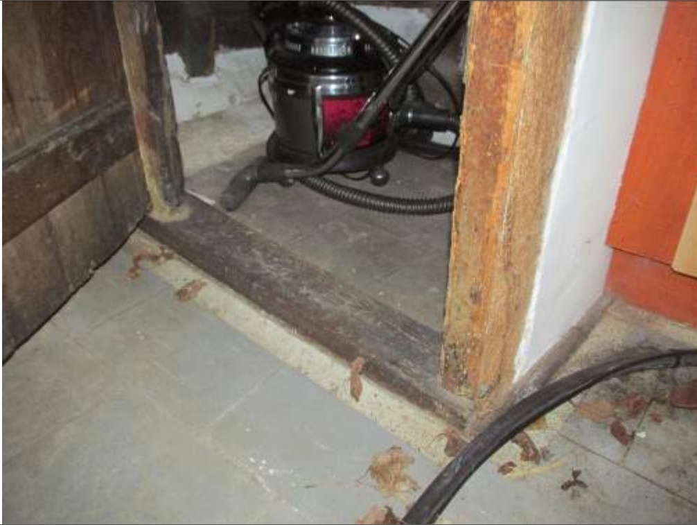
Photograph 19 – Internal base to stairs to be re-supported on new limecrete slab
