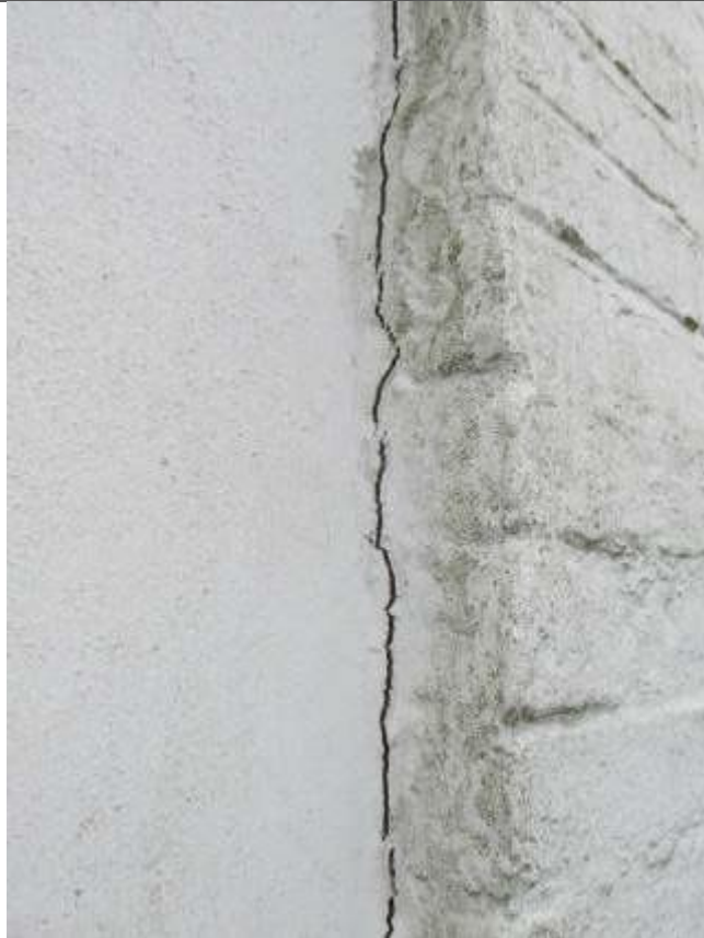
Photograph 10 – End lean-to bulge to north face due to rotation
