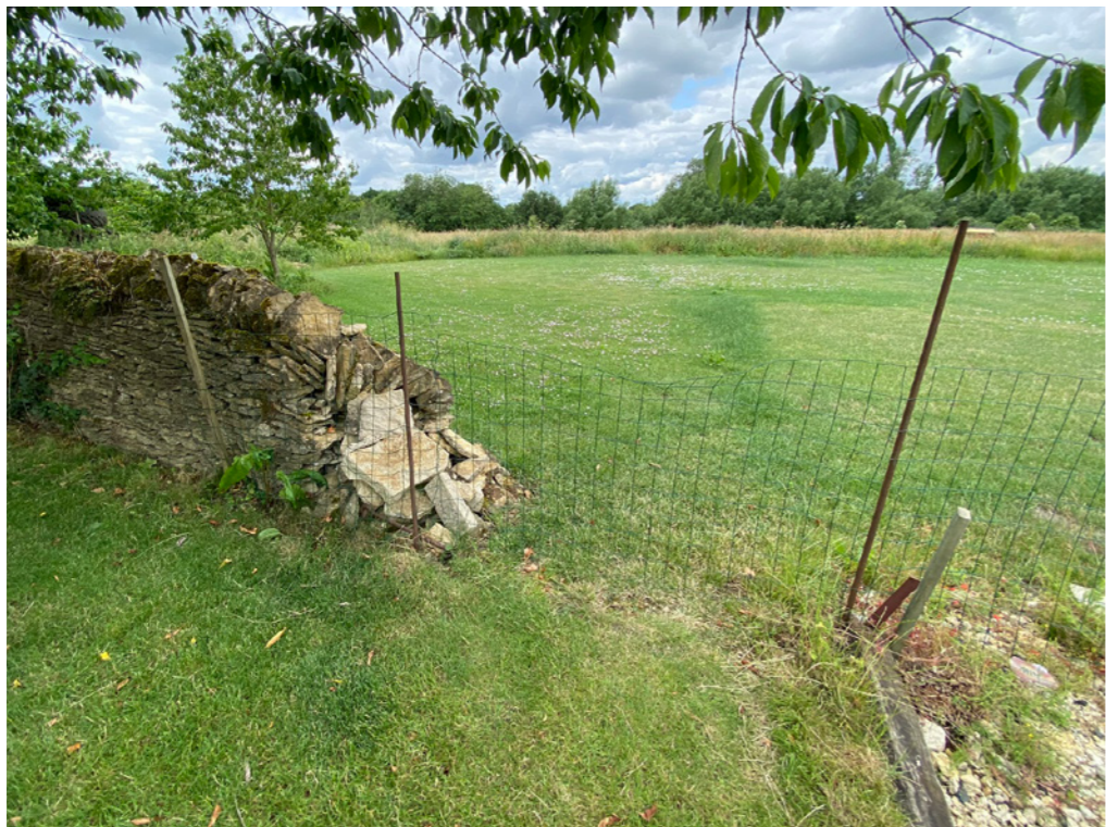
Original western boundary 0.9 m tall dry stone wall. End of wall to be repaired. Pig mesh to be replaced with post & rail timber fence. Work to be completed in 2024
