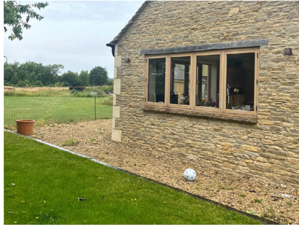
Footpath - current hardcore to be replaced by Cotswold chippings. Work to be completed in 2024
