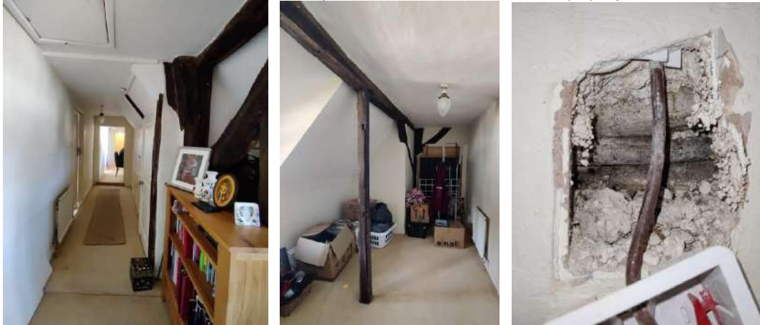
Figure 34 First Floor 18 th century timber framing in historic core Figure 35 First Floor 18 th century timber framing in historic core Figure 36 First floor wall opening up showing horizontal branches in situ in historic core
