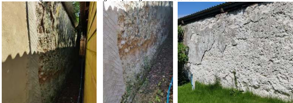
Figures 96 – 98 Views of poor historic wall condition
