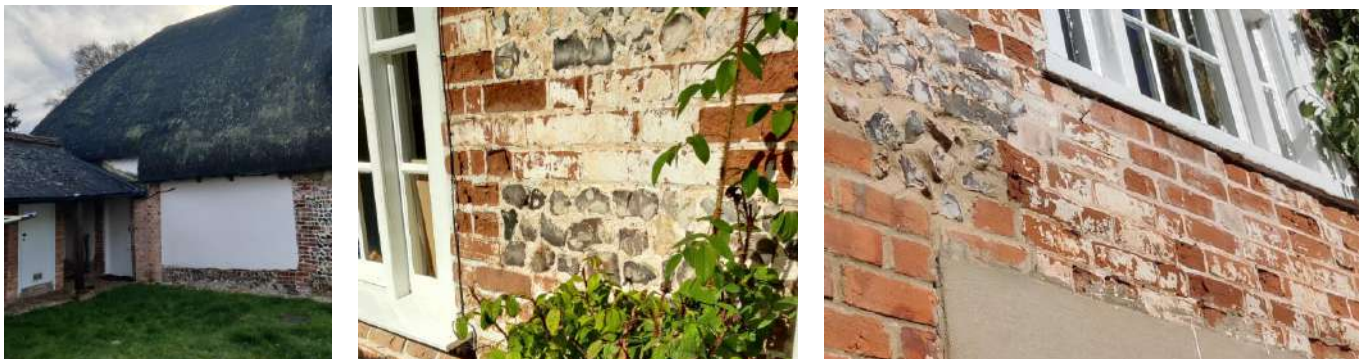
Figure 145 Cement rendered area on north elevation Figure 146 & 147 Areas of blown faced brickwork
