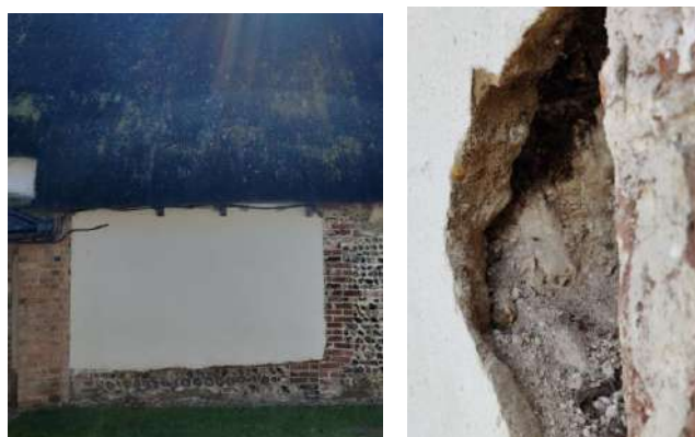
Figure 119 Image of area of wall for new fire door Figure 120 Scope survey of missing area of cement render showing poor condition fabric behind
