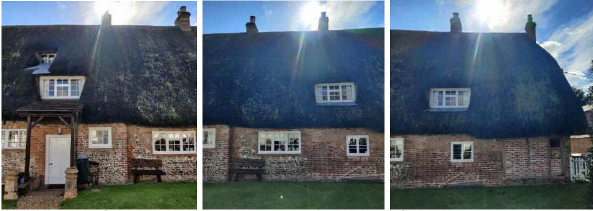
Figure 87 Early 18 th century core of the property. Flint walls with large areas of 20 th century flint and brick replacements. Figure 88 Early 19 th century section of the property. The flintwork matches the majority of the north elevation suggesting a period of refacing assumed 19 th century. This area has large areas of 20 th century flint and brick replacements. Figure 89 Early 19 th century section of the property. Complete refacing in 19 th century Flemish Bond brickwork. Figure 90 Early 19 th century extension of property. Timber framing with Flemish bond brick infill panel.
