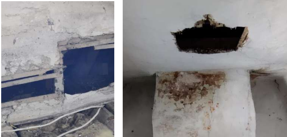
Figure 143 & 144 Missing areas of lath and plaster and water damage in Attic space
