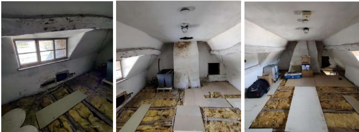
Figures 127 – 129 Images of Attic including areas of lost and damaged fabric
