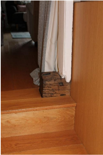
Photograph 4: doorway to living room showing protruding soleplate
