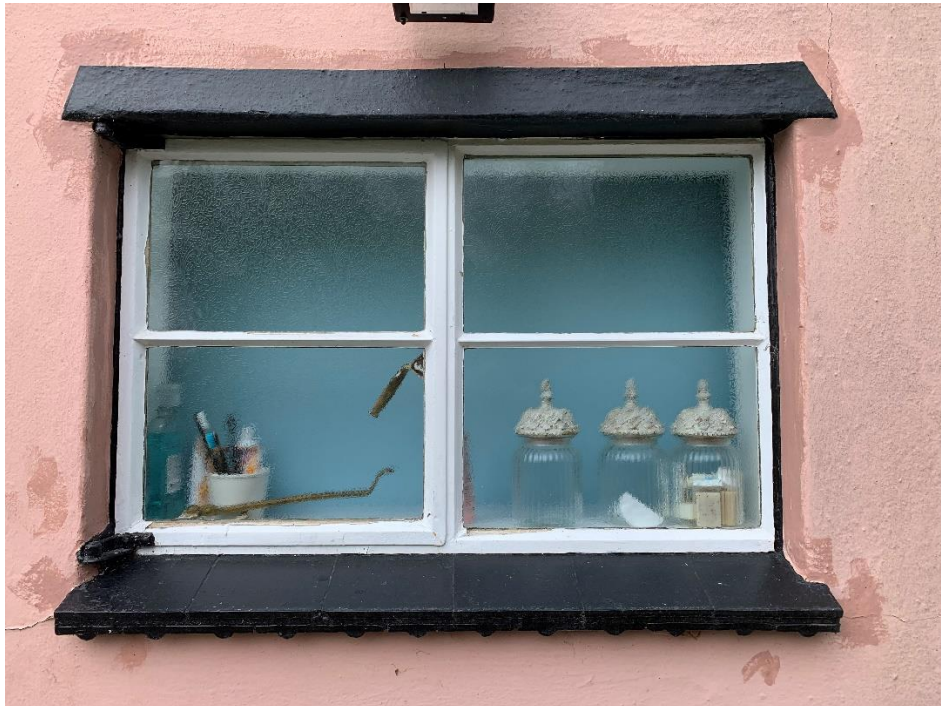
Metal framed and single glazed with timber pentice board and creasing tile cill
