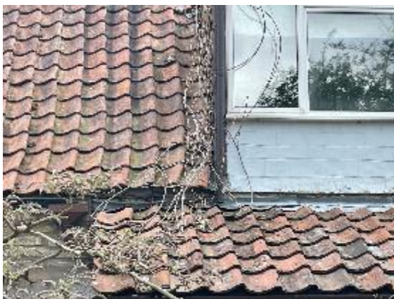
Plate 3: Gap between lead flashing and tile
