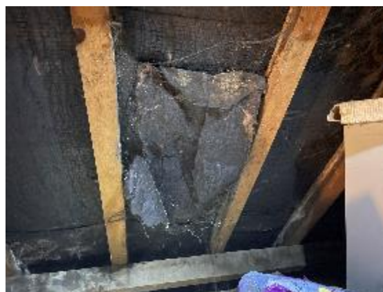
Plate 6: Gap in internal roof lining
