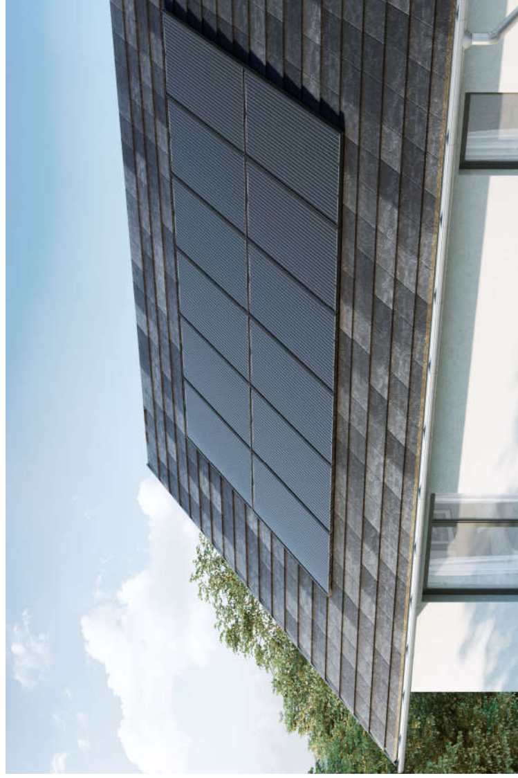
Image B – PV solar panels to rear
