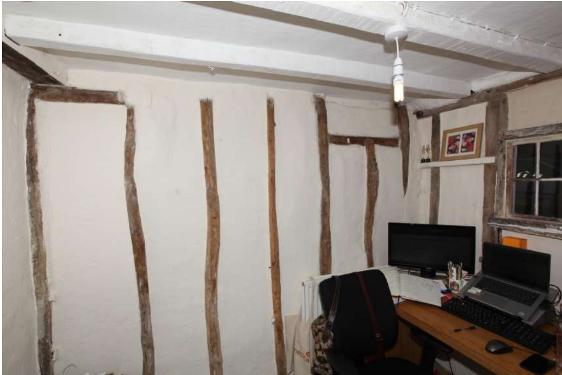
Illus. 13. The ground-floor partition to the west of the former pantry in illustration 12, with its blocked door on the right and the partition adjoining the stair lobby in illustrations 10-11 on the left. These are the only original internal walls to survive on the ground floor. The ceiling consists of common joists tenoned to a central axial joist on the left which is in turn supported by a short rail nailed to the studs. The same lintel presumably supports the narrow axial joist of the living room ceiling, which is constructed differently (with its joists resting on rather than tenoned to the axial joist).
