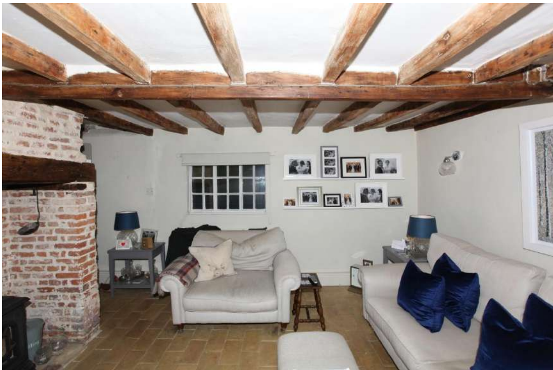
Illus. 8. The front wall of the well preserved eastern cottage showing the 3.5 m length of its principal room with the position of the blocked entrance door to the right of the window in illustration 9. The ceiling is original to the structure and unusually consists of re-used timbers with lath nails in their sides which span the walls and are lodged upon rather than tenoned to a central narrow-sectioned axial joist of pine.
