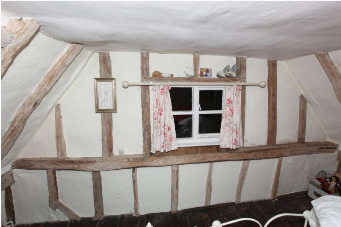
Illus. 27. The intact original studwork of the western gable with the top of a nailed diagonal primary brace visible to the left.
