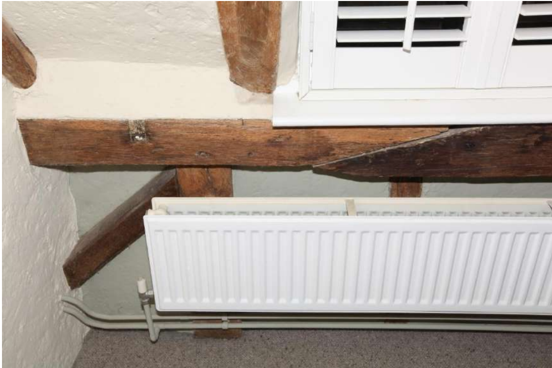
Illus. 23. A detail of the wall framing in illustration 20 showing a crude, diagonally splayed scarf joint with a re-used section of roof-plate on the left containing a dovetail joint for a tie-beam that is not matched in the opposite plate to the rear. The straight, diagonal primary braces interrupt the vertical studs and are nailed rather than pegged to the frame. These features all indicate a date towards the end of the framing tradition.
