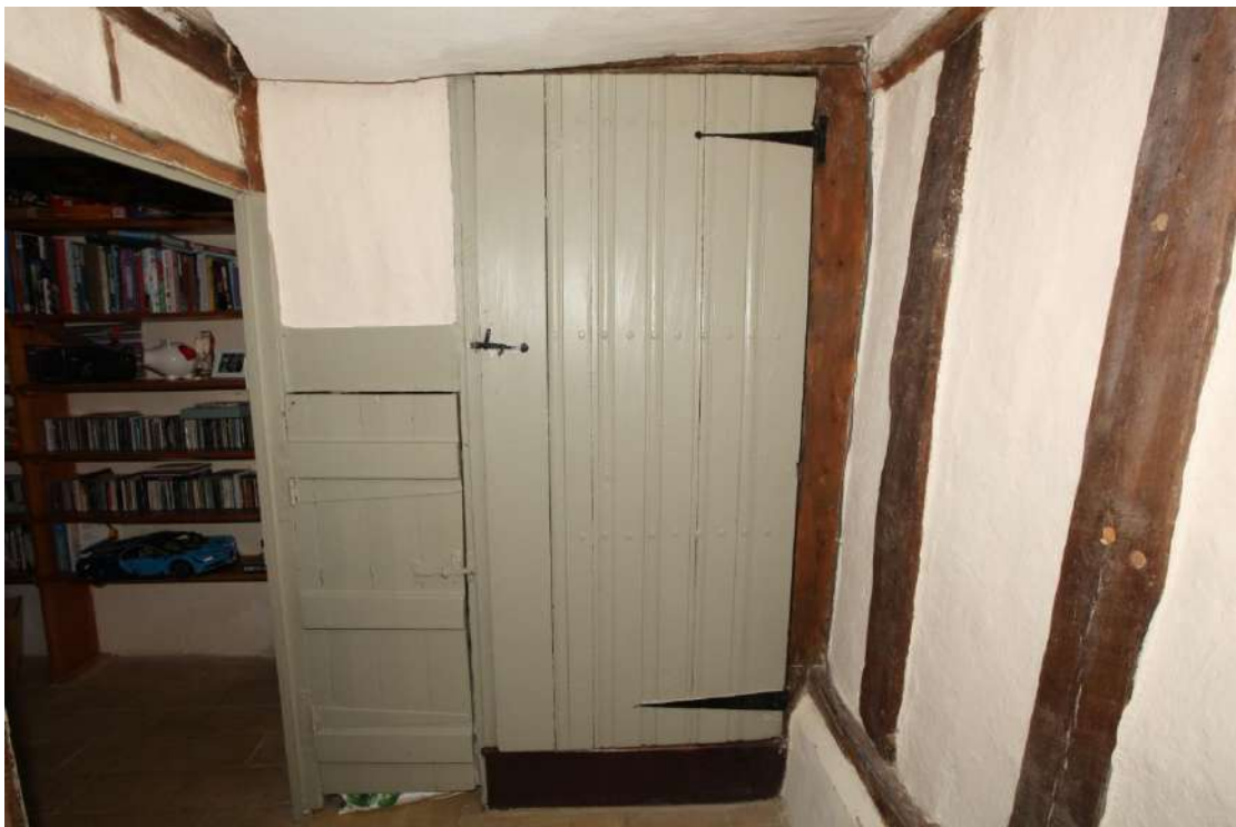
Illus. 10. The door to the original stair in the south-eastern corner of the building with the inserted entrance to the study on the left (originally a pantry). This door is a good 17 th century example consisting of moulded planks, but was extended with a plain board on the left when it was re-used in its current position.
