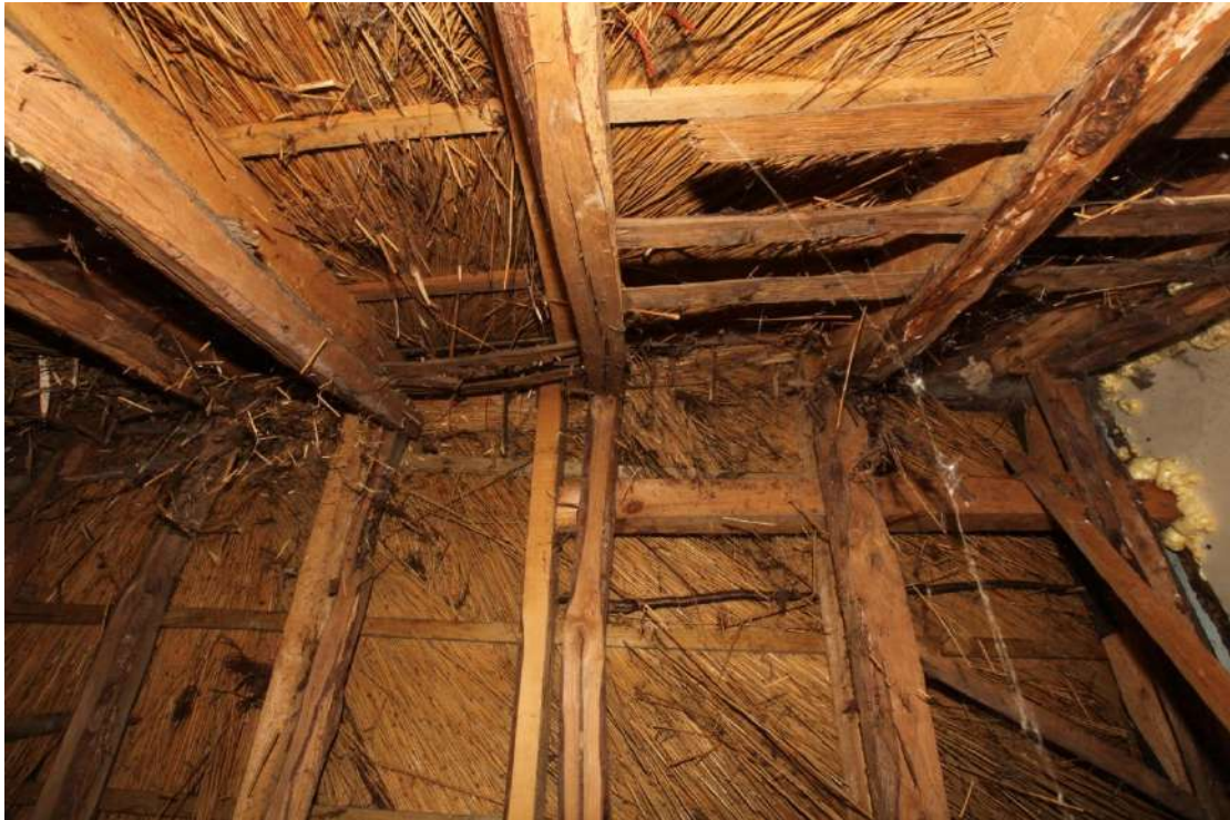
Illus. 21. A detail of the roof showing the plasterboard-clad eastern gable on the right. The size of the original rafters varies considerably, with some like those on the left no more than 2 inches square at the apex, but all are neatly pegged where they overlap.
