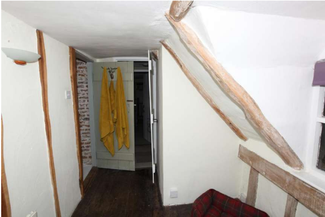
Illus. 25. The bedroom above the western hall/kitchen looking east towards the chimney and the partition enclosing the modern stair. The wall to the left is a modern insertion consisting of unpainted studs intended to replicate the originals and now forming the southern wall of a bathroom.
