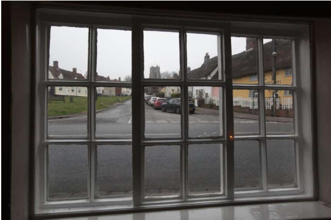
Illus. 9. A detail of the good 19 th century horizontal sash window in the front wall of the eastern living room, with the famous view of the green beyond. These windows may well be contemporary with the building.
