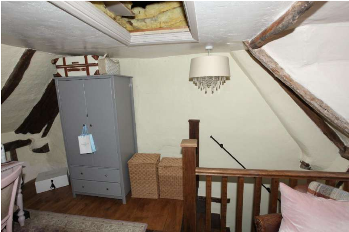
Illus. 19. The eastern internal gable of the structure on its upper storey. The timber-framed walls were simply built against the earlier cottage with no separate gable of their own. The projecting, weathered ends of the neighbouring building's roof-plates are clearly visible to left and right, having form an external wall prior to the addition of The Old Thatched Cottage.
