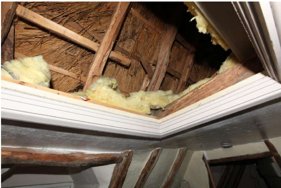
Illus. 20. The original clasped-purlin roof structure survives intact (as seen from the easternmost bedroom in illustration 19). In contrast to the external walls there is no evidence of re-used timber, but many of the rafters are unusually slender and new softwood rafters have been inserted alongside.
