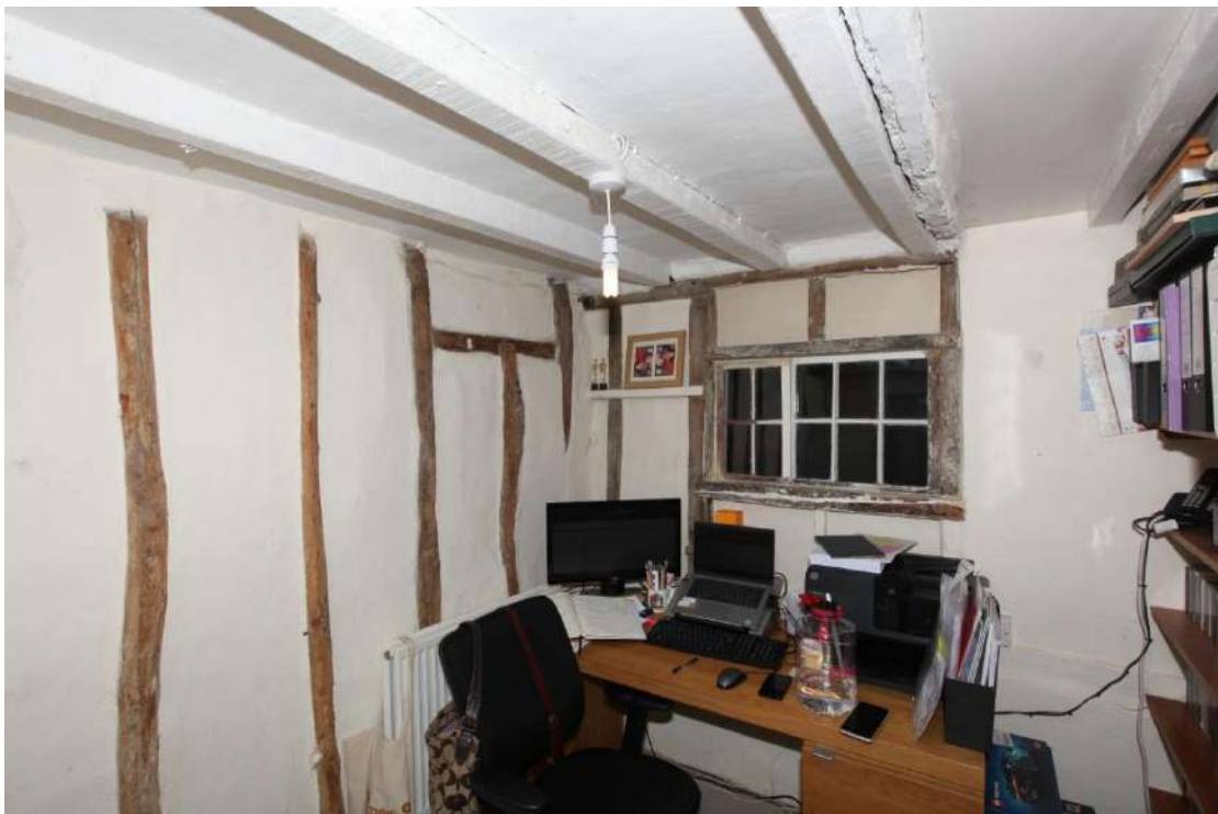
Illus. 12. The study in the north-eastern corner of the building, lit by another horizontal sash window that fits the original wall framing. This room would have operated as a pantry and general storage area, and was directly linked to the main room by the blocked door to the left of the window. This door was later blocked by a short stud nailed to the original door lintel.
