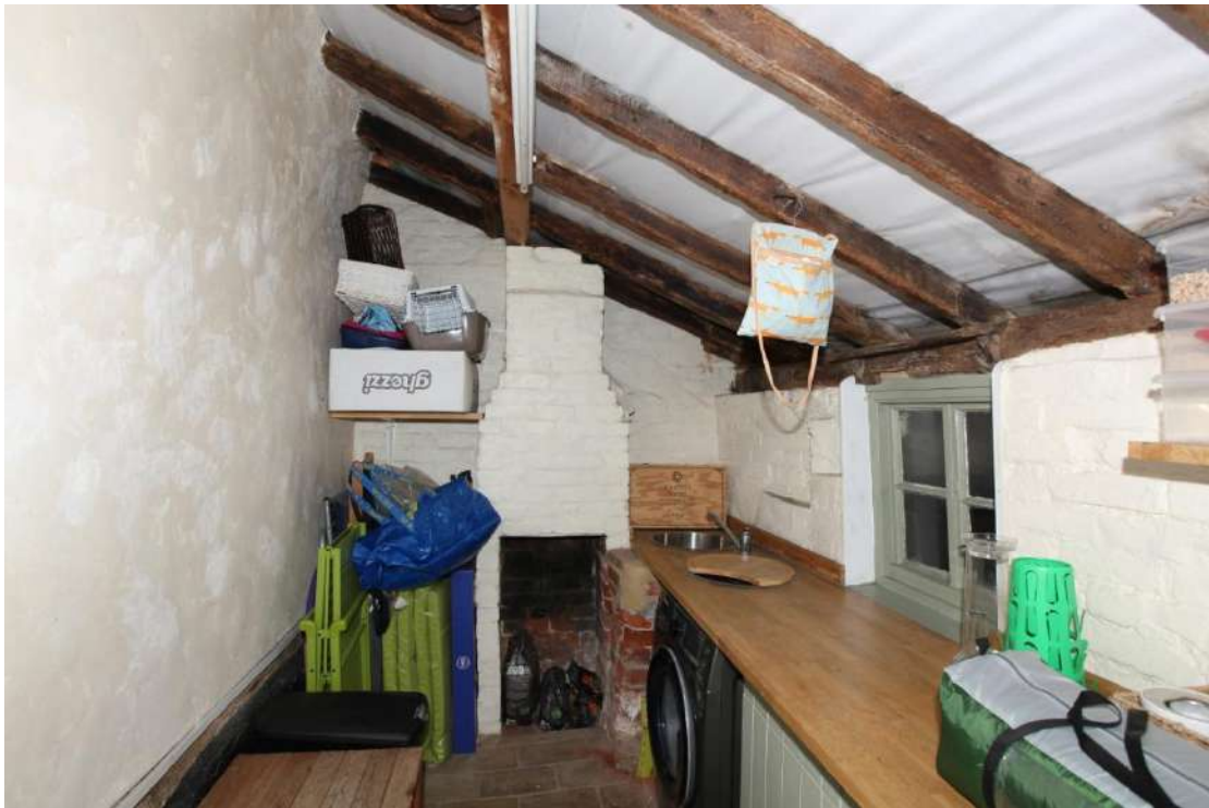
Illus. 4. The interior from its western entrance of the rear lean-to showing its narrow fireplace with a hot water copper to its right. The main chimney has been truncated below the roof and an area of disturbance in the brickwork to the right of the copper suggests it once possessed a separate flue of its own.
