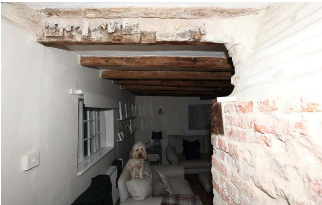
Illus. 14. A detail from the west of the nailed notches for the missing original partition studs between the two cottages, with the remains of wattle-and-daub infill above. The partition remains place on the first floor (to the left in illustration 22).
