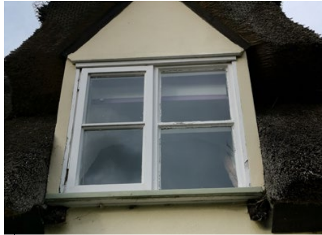
All timber windows noted on drawings to be replaced with slimlite glazing.
