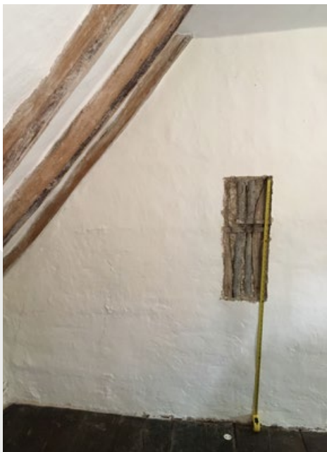
Investigation works in area of proposed relocated door, indicating no tie beam.
