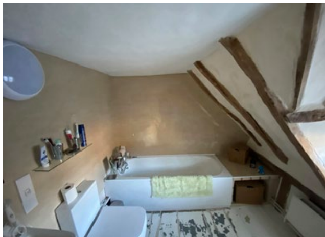
Existing bathroom to be relocated to rear of property. New opening created on far side wall.
