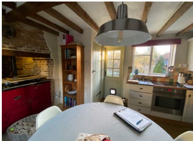
Modern internal partition to staircase to be removed. Back door to be re-hung to allow for opening inwards.
