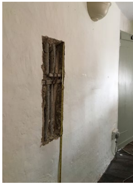
Investigation works in area of proposed relocated door, indicating no tie beam.
