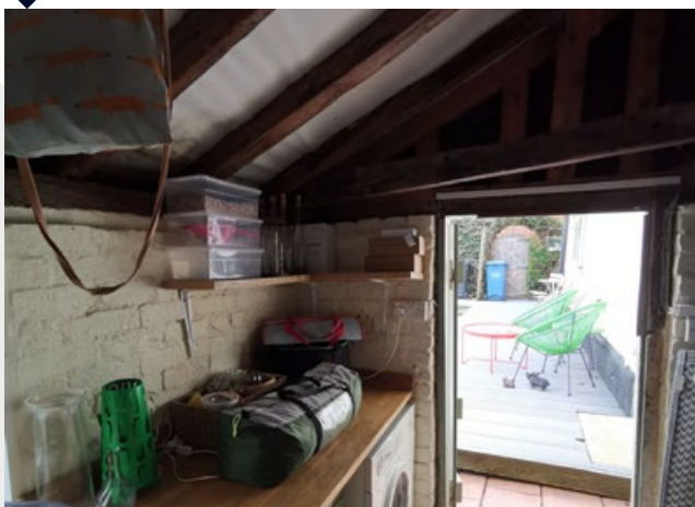
Internal view of later addition, external walls to receive insulation on internal leaf. Existing roof to receive insulation.
