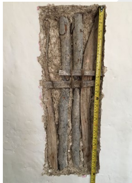
Investigation works in area of proposed relocated door, indicating no tie beam.
