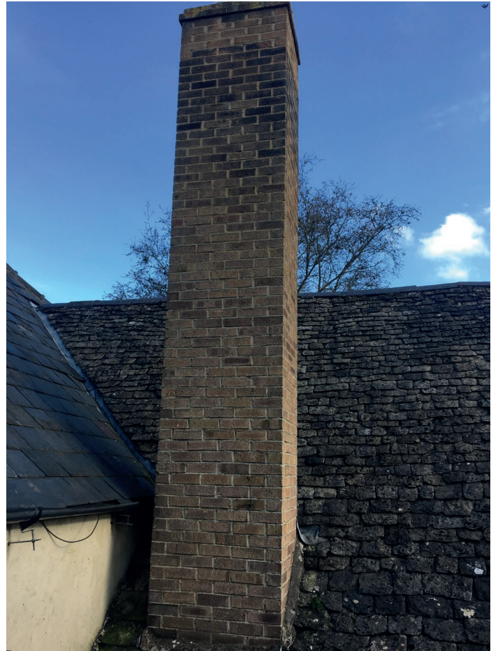
The tall modern chimney to the easternmost building at the rear of the Bull. Unstable it is proposed to be removed
