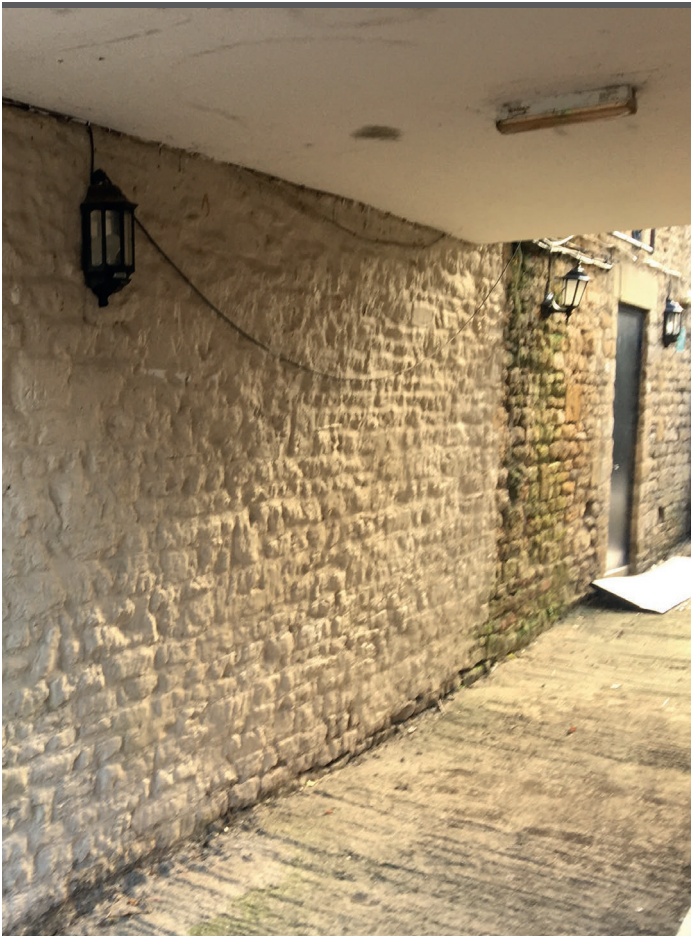
The carriageway which connects the Bull's yard to that of the Post Office. The doorway to be filled to the right of the image
