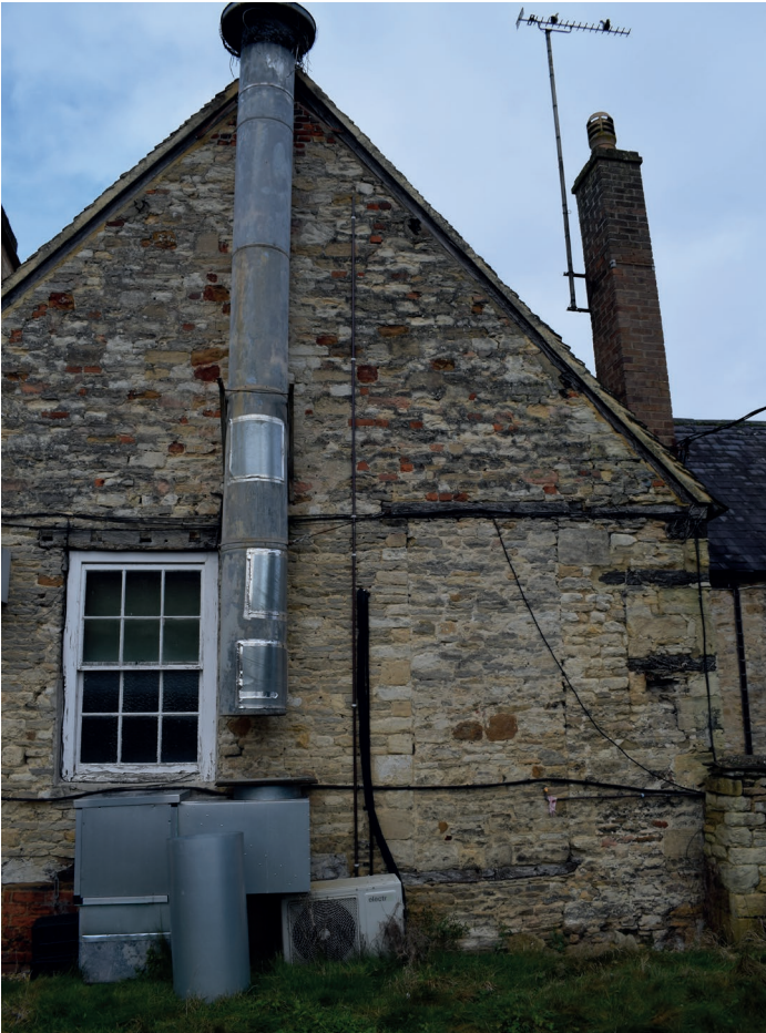
Current plant equipment to be relocated from the Post Office yard
