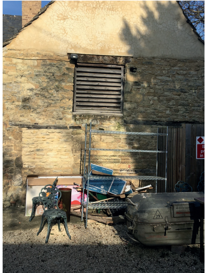
The end elevation of the easternmost outbuilding viewed from the postoffice yard. The timer louvre is to be replaced with a window and a window opening created to serve the ground floor below
