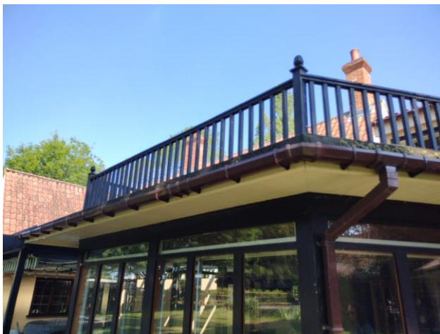
Photo 9: closer view of the roofline on the existing sunroom to the south of the property.
