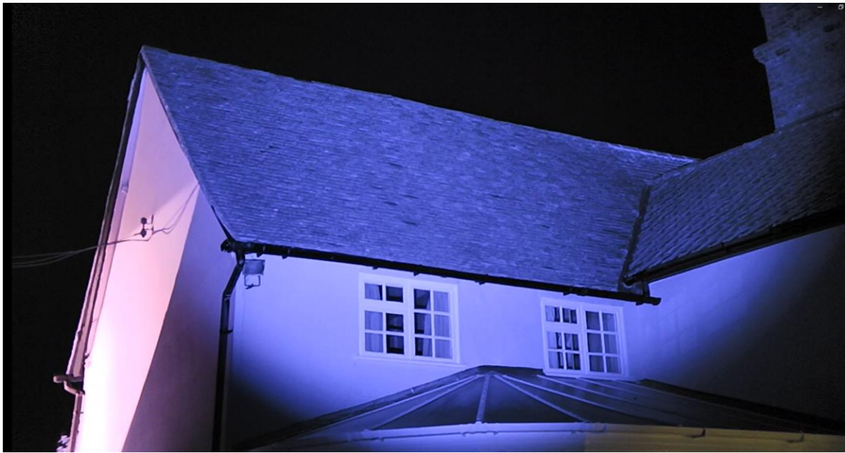
Plate 3.1: SiOnyx Aurora with Nightfox XB5 illuminators – SW of House - 17.05.23 (end of survey).
