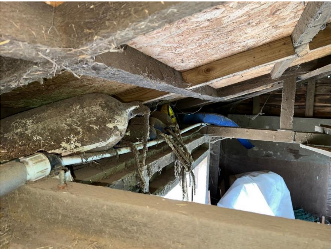
Photo 16. View of storage area above soffit in building 1. Taken from within unit B1d.
