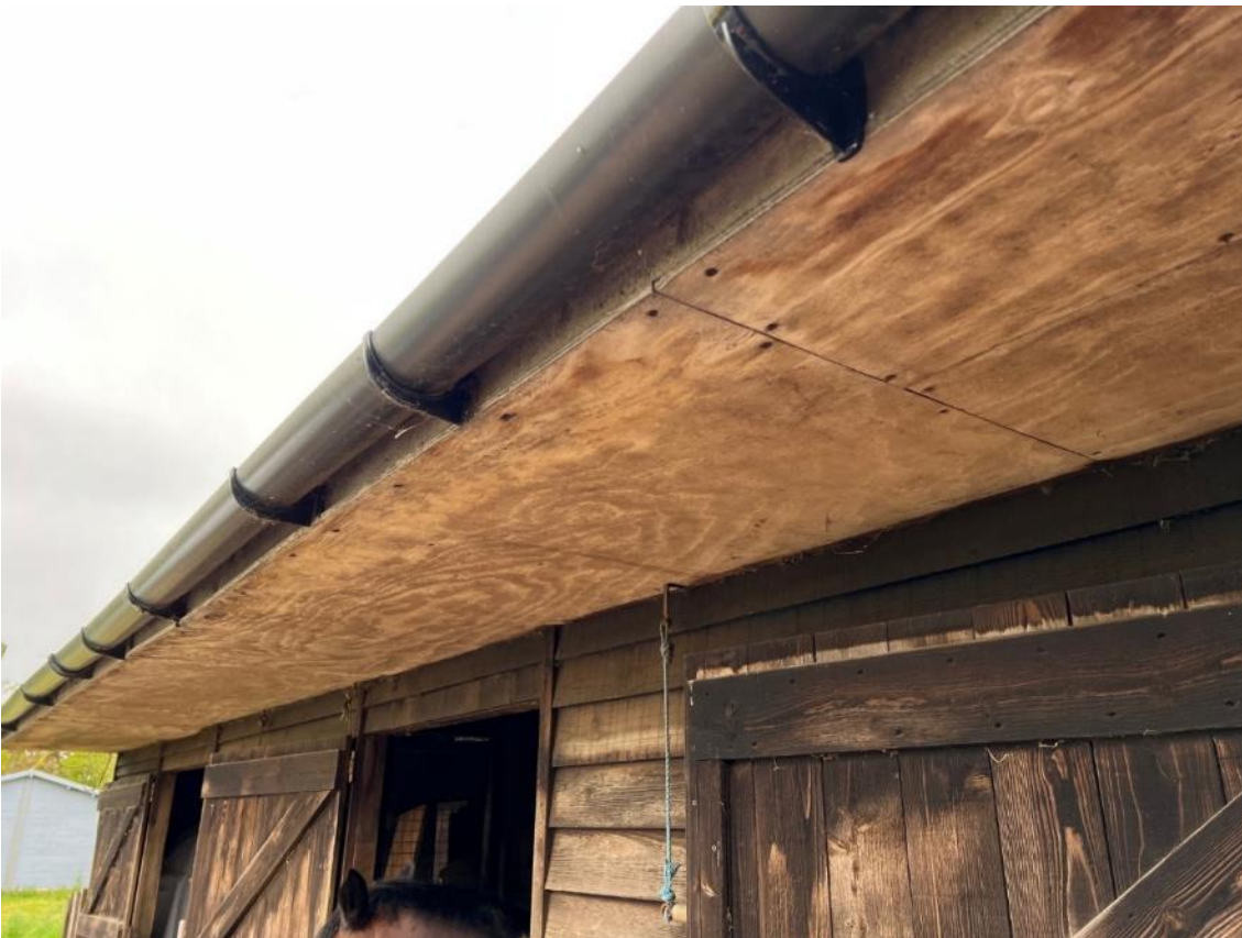
Photo 10. View of plywood soffit on the stables, building 1. Above unit B1c and B1d.
