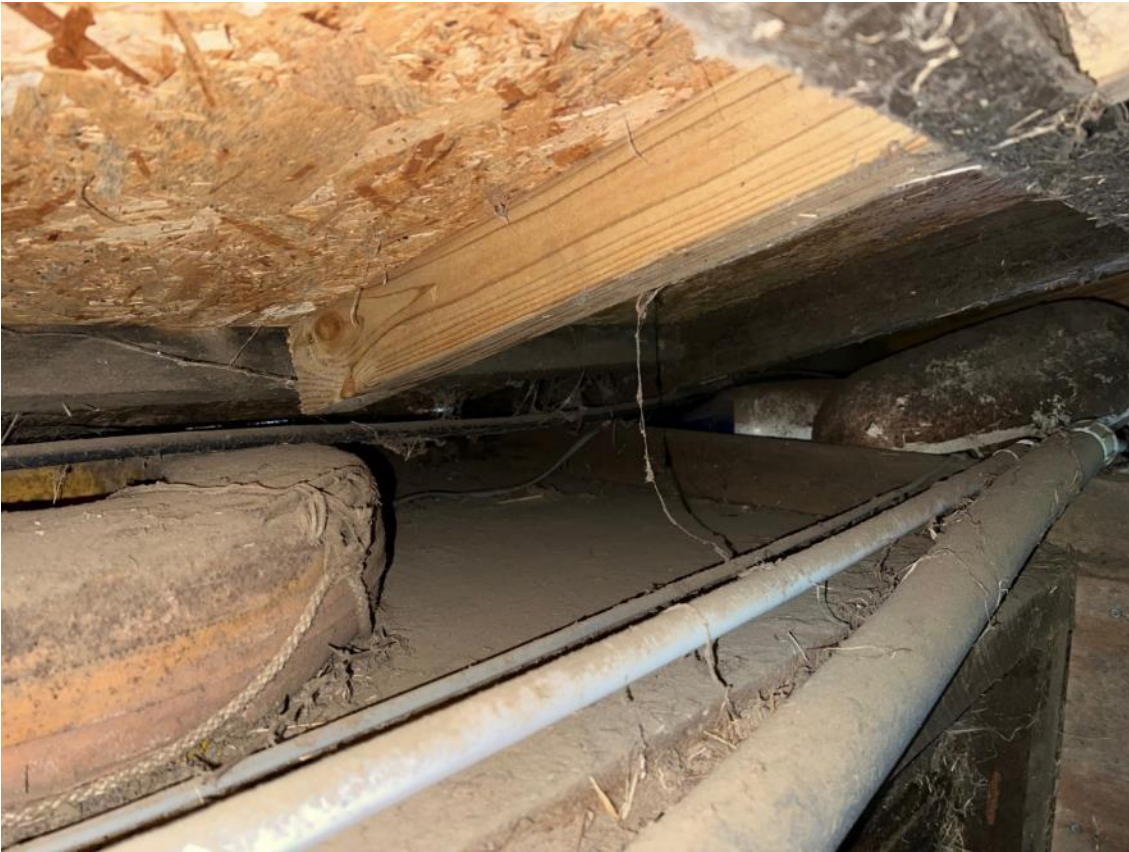
Photo 17. View of storage area above soffit in building 1. Taken from within unit B1b.
