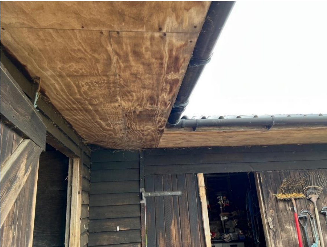
Photo 9. View of plywood soffit on the stables, building 1. Above unit B1a and B1b.
