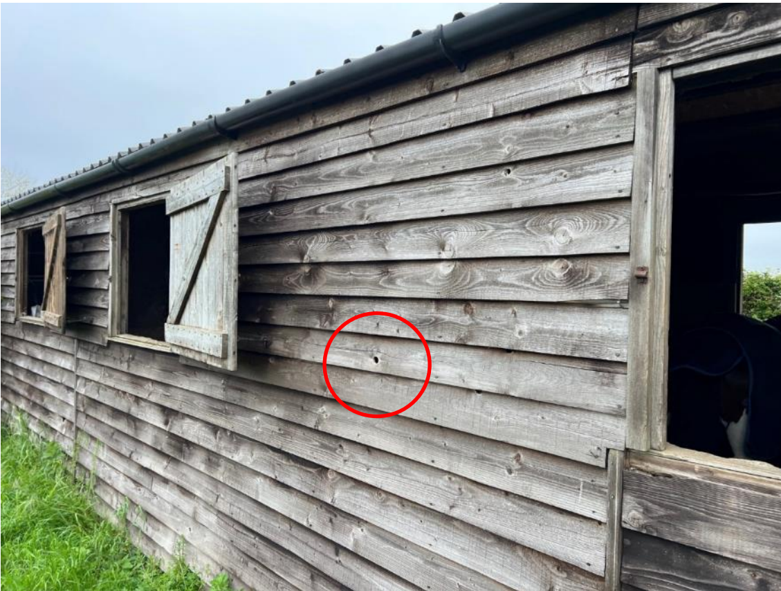
Photo 7. Rear of the stables, building 1. Small rot hole, where bluetit entered as identified by red circle.
