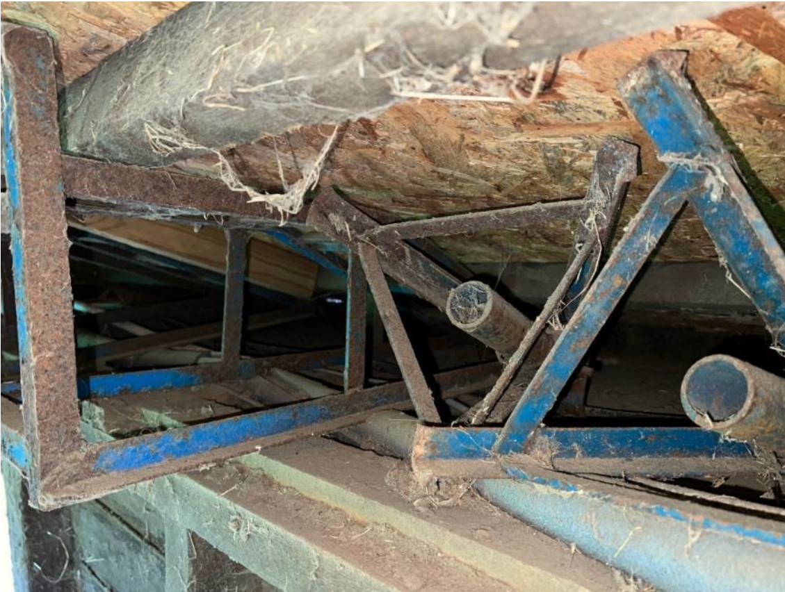
Photo 15. View of storage area above soffit in building 1. Taken from within unit B1c.
