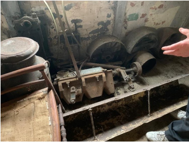
An original water wheel bucket is stored on the ground floor. A replica of this bucket has been made up in cast iron and is currently stored in the building.
