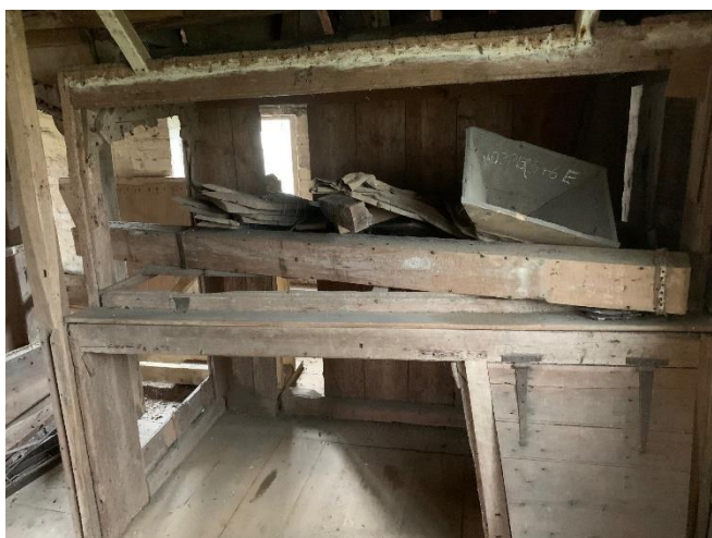
The dresser will be retained in the refurbishment plans and relocated to allow passage of the new staircase
