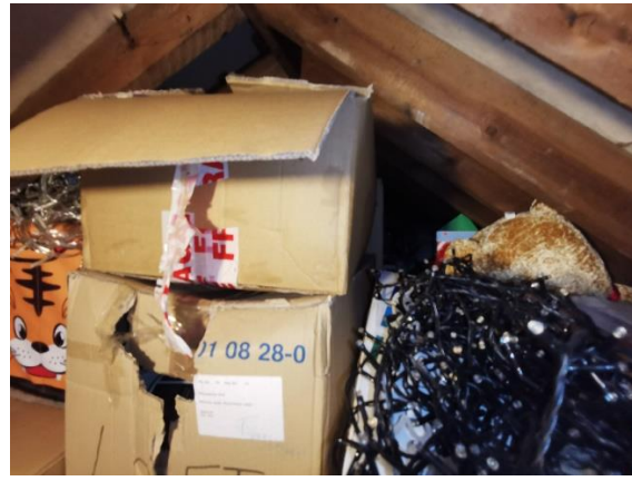
Limited accessibility due to storage use of the loft space.
