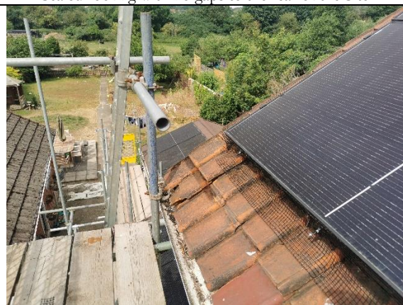
Minor damage to tile at the rear of the Site
