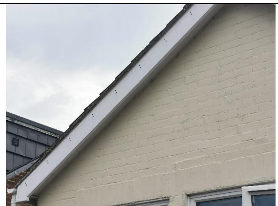
Sealed barge boards with no ingress points.
