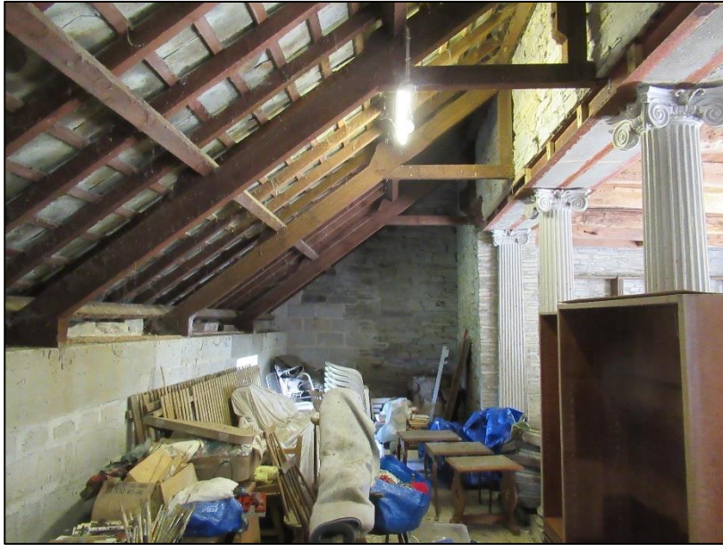
C20 extension built on to the north west side of the original stables.
