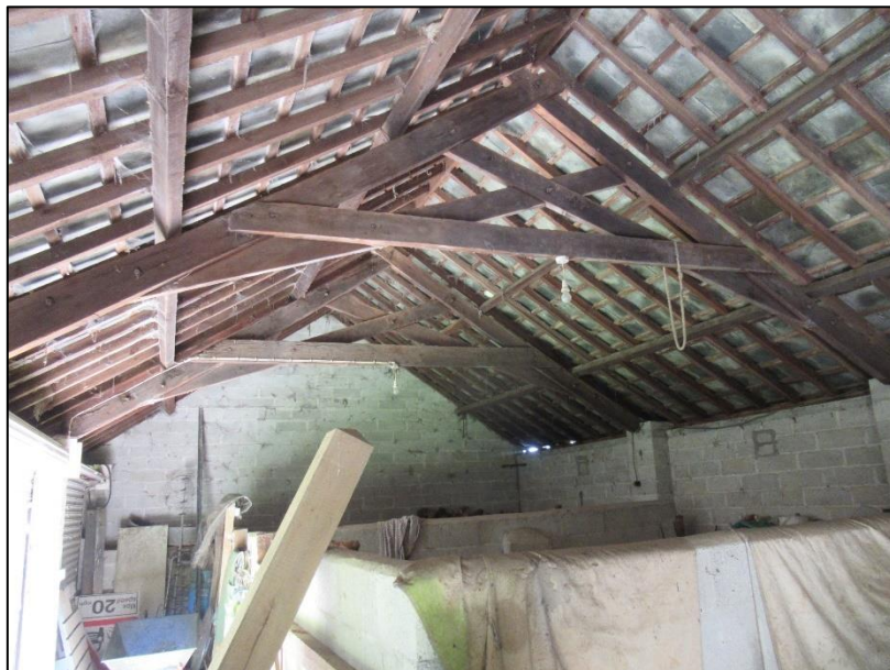
Truss and purlin roof structure supported on concrete block walls, in turn generally built off earlier stone walls.
