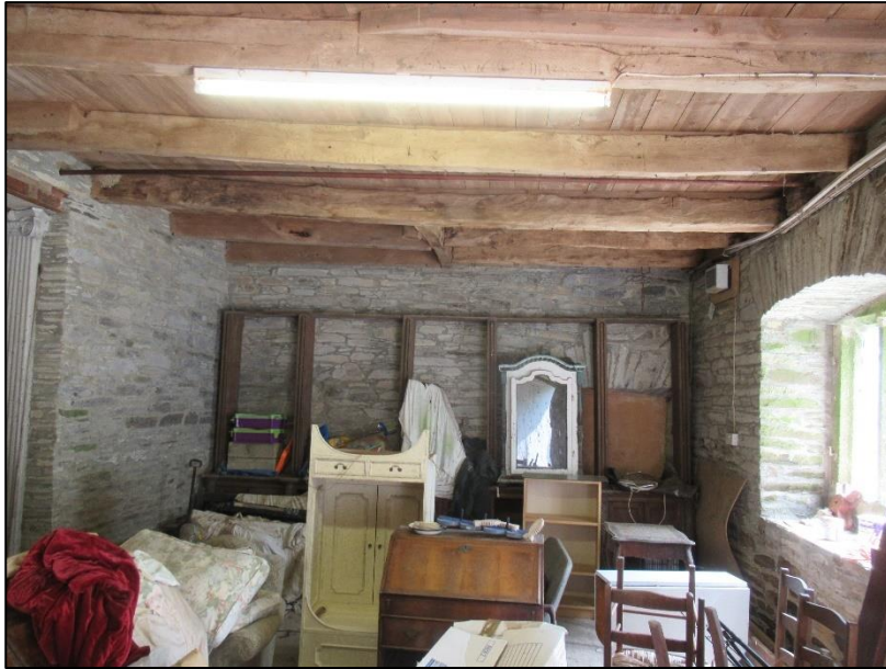
Existing first floor structure with original oak joists spanning the width of the building supporting later boarding.
