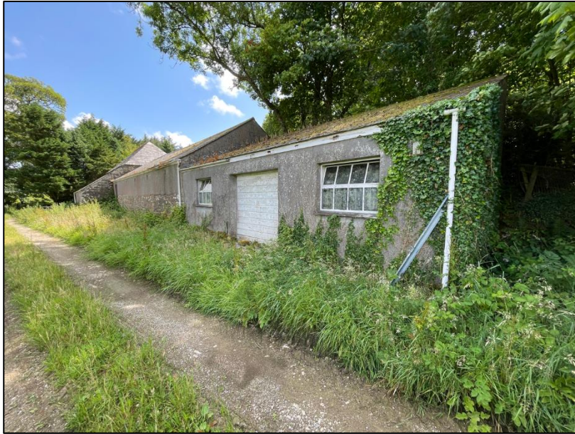
Modern barn or garage sited at the western end of the complex.
