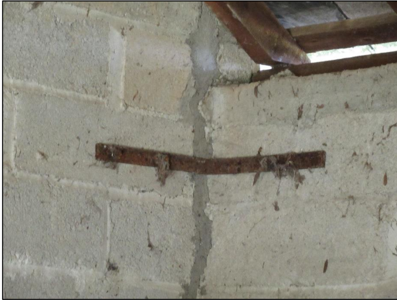
Previous strapping introduced to western corner of the barn with previous cracking infilled. No serious evidence of recent significant movement in this area.
