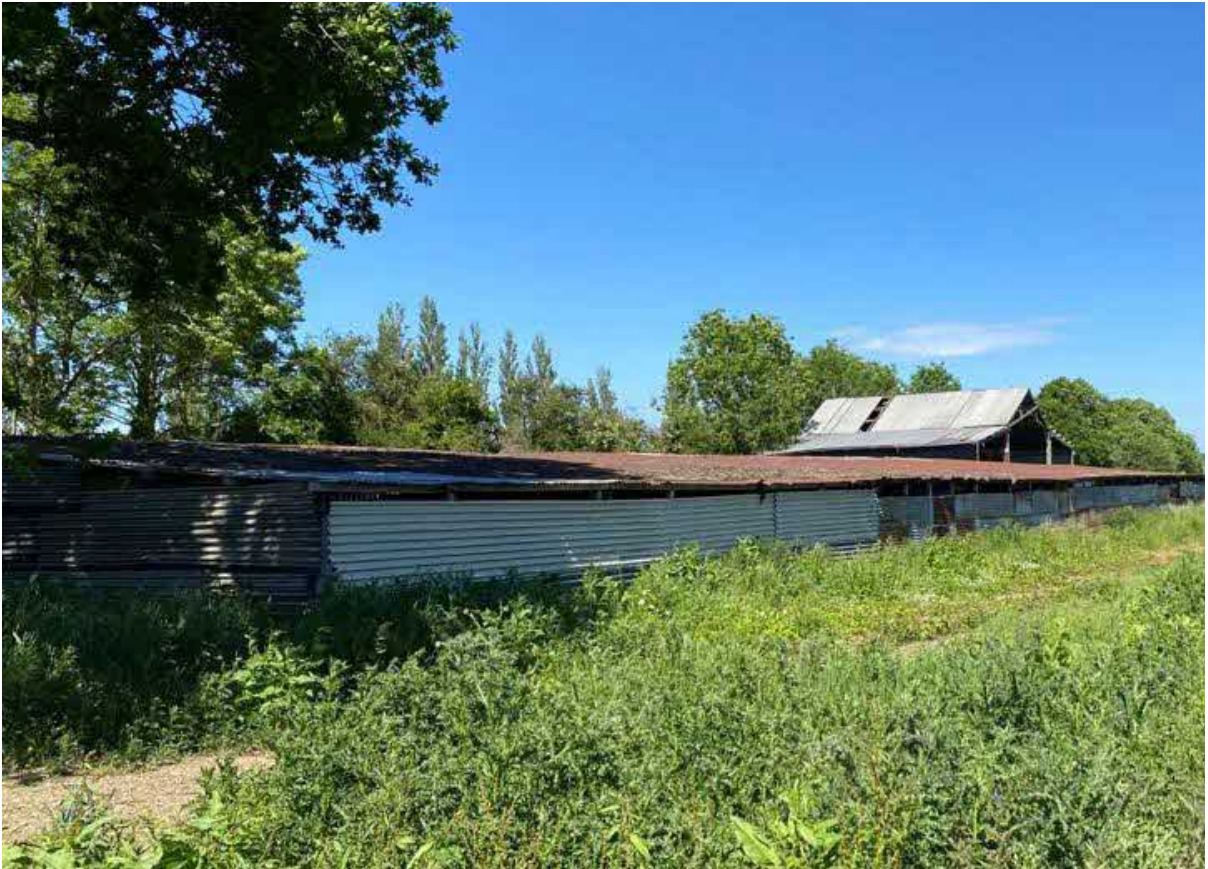
Photo 8. Exterior of the Turkey Barn (B3) to be partially demolished, taken at southwest corner of building looking northeast, with Barn 2 (B2) in the background
