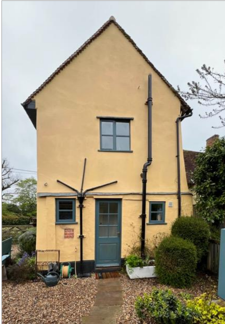
Fig.9 East gable end elevation to Coflee showing underbuilt ground floor in brick (with cover lead flashing and modern casement windows and door) and a panel of investigation of the rendered ground floor exposing red Imperial brickwork in lime mortar
