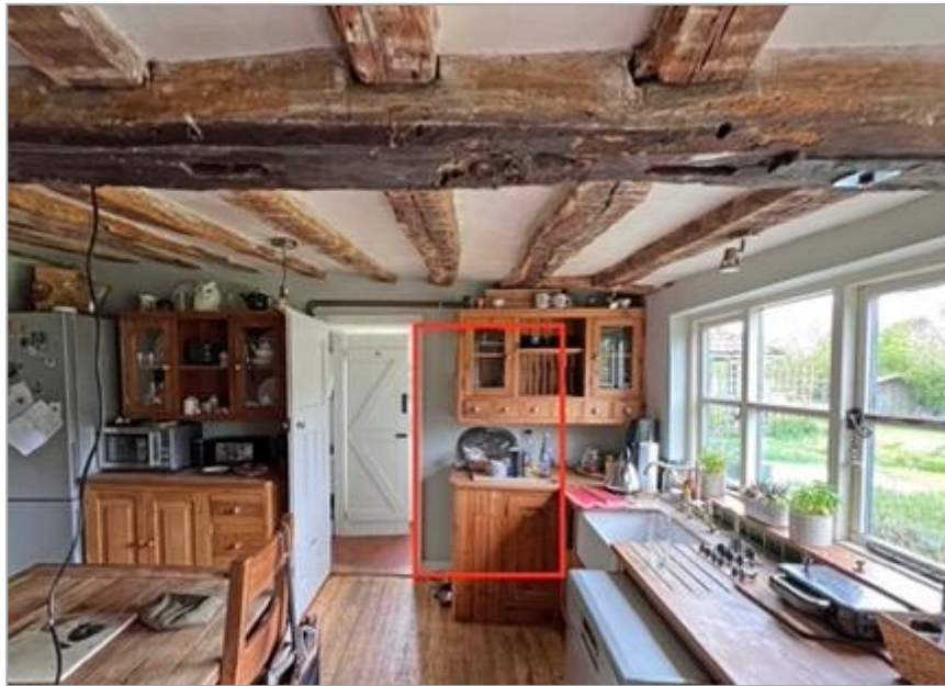
Fig.10 Kitchen facing east with proposed enlargement of the plastered brick wall indicated in red. Note the modern kitchen and WC doors. Ceiling joists unaffected by the proposals.
