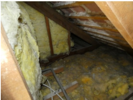
Side void: Partially unlined and filled with fibreglass insulation
