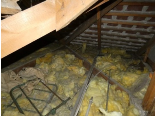
Main roof void: Unlined and partially parged slates
