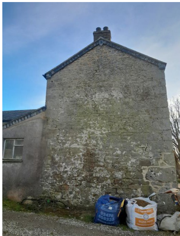
Fig. 7 Gable End revealing earlier bag rubbing
