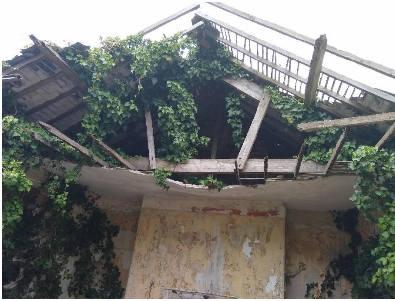
Figure 19 Showing the remains of the roof and first floor ceiling in C19 house
