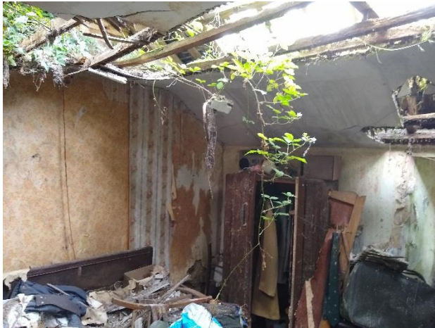
Figure 13 Collapsed first floor ceiling in C17 house
