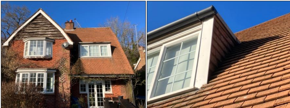
Photographs 2 a (left) & b (right). a) View of the main house from the eastern aspect where the new ground-level infill extension is proposed. View of wooden cladding to the top of the building. b) View of the window feature located in Photograph 2a (left of image). View of hanging tiles with some gaps noted to the northern aspect. Hanging tiles noted to both aspects of the window.
