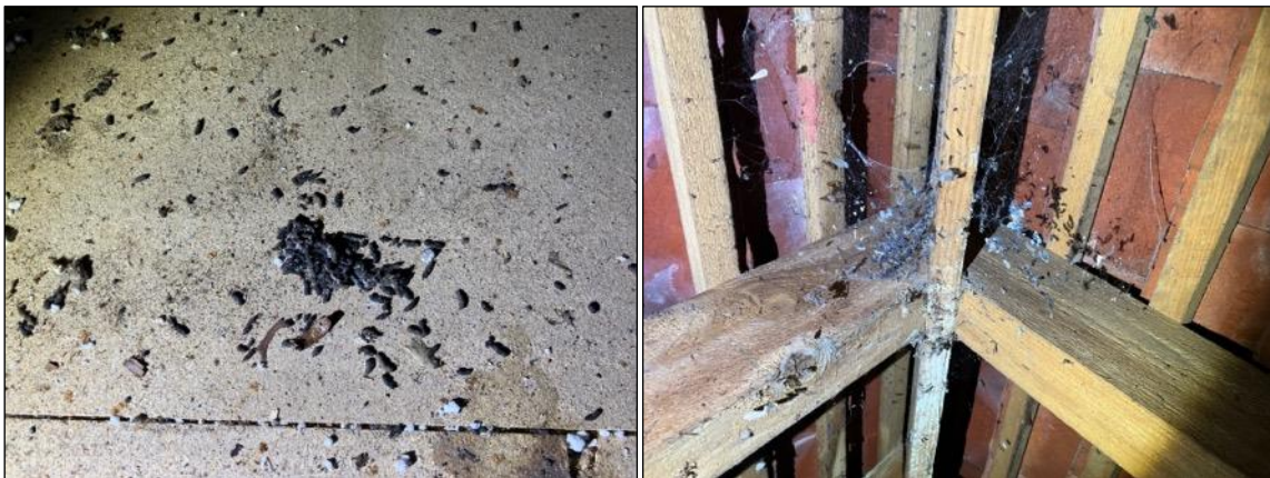
Photographs 4 a (left) & b (right). a) View of long eared droppings from the first loft space. b) View of droppings caught by cobwebs to the apex of the first void. Note the lack of roofing felt within this loft void providing increased access and egress points across the space.
