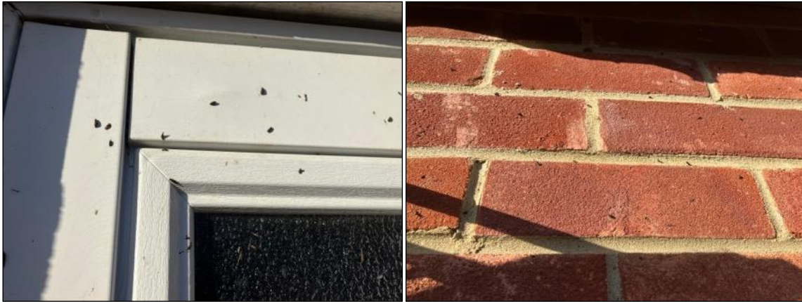
Photographs 6 a (left) & b (right). a) View of the right garage door as seen from Photograph 5a, view of several bat droppings noted contrast against the white door. b) View of the brick work below the wooden cladding with view of bat droppings again.
