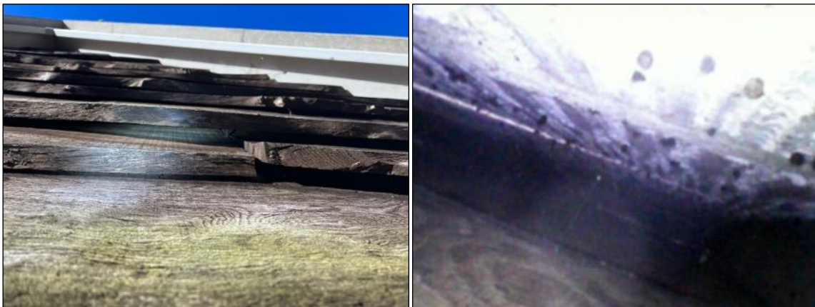
Photographs 7 a (left) & b (right). a) View of the wooden cladding as illustrated in photograph 5a clear gaps can be seen across the boards. b) View of bat droppings from within the cladding as indicated in photograph 7a, image taken using an endoscope.
