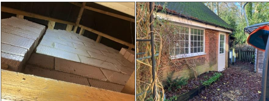
Photographs 8 a (left) & b (right). a) Internal view of the garage unit facing the breezeblock construction (backing of the wooden cladding). This section is well intact and any roosting bats within the cladding will be restricted within this aspect unable to migrate to other aspects or the internal area. b) View of the northern aspect of the garage block, some slipped tiles are noted although infrequently. The open space within the garage is considered to be of lower temperature than that of surrounding habitats and roosting features.
