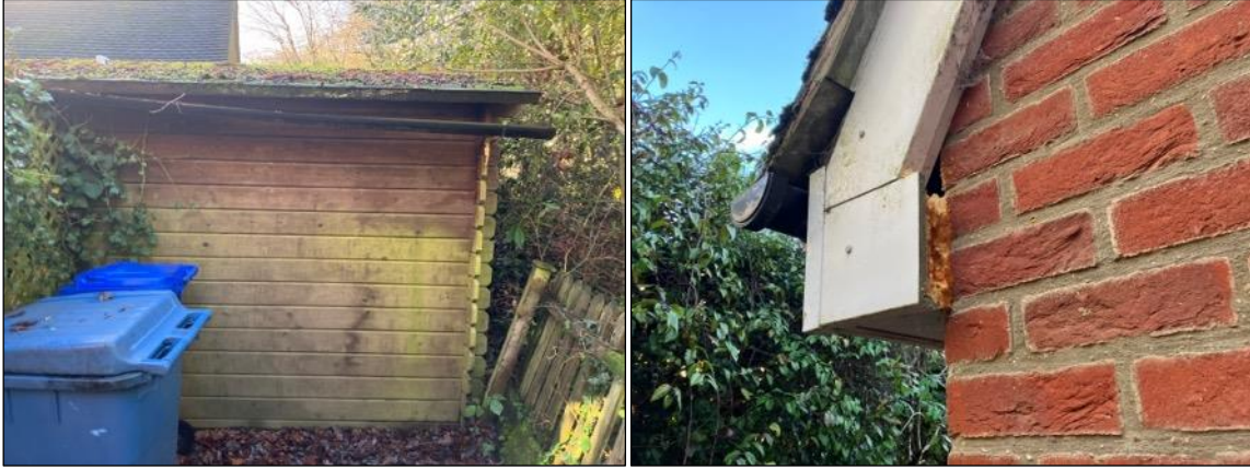
Photograph 9 a left & b right). a) View of the shed located to the western aspect of the site, image taken from the northern aspect. b) View of the main building to the north western aspect of the site, view of potential access/egress point visible to the fascia.
