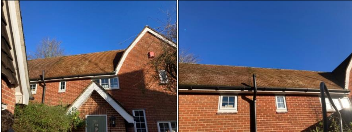
Photographs 1 a (left) & b (right). a) View of the main house from the southern aspect with view of the main door to centre of image and lifted tiles noted. b) View of the main house from the southern aspect with views to damaged/lifted tiles.
