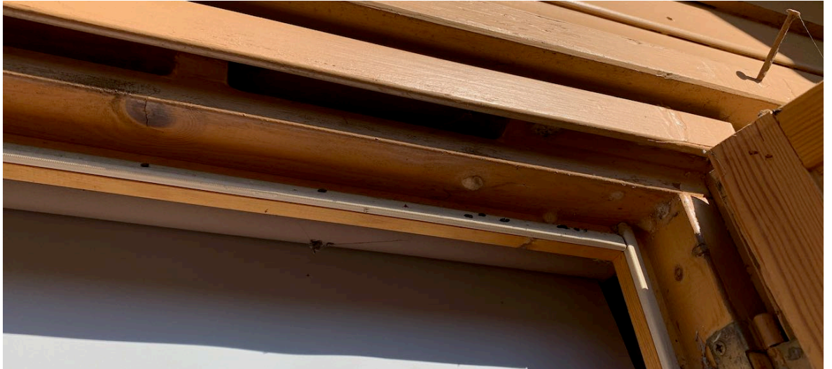
Photograph 3. Common Pipistrelle droppings around window frame (with broken vent visible above)
