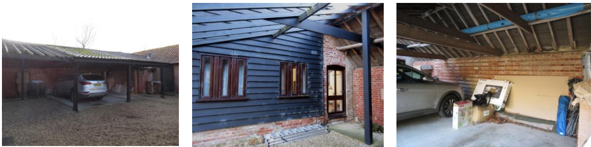
Left: cartlodge looking SW; Centre: interior of cartlodge showing existing door into playroom attached to main barn; Right: looking NE showing banded brickwork in S wall
