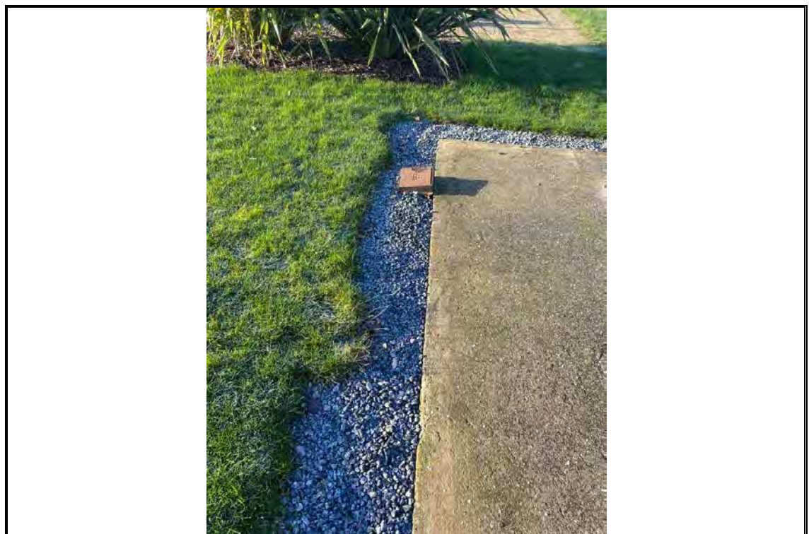
Photo OE/1702/1048 R1 PF2 – P02 – 0.3m wide, 0.2 deep – gravel drainage at side of parking area
