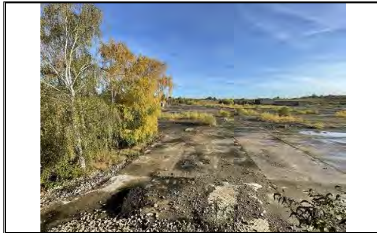
Photo OE/1702/1048/R1/P10 – General view of site and exposed concrete slabs – looking southwest.
