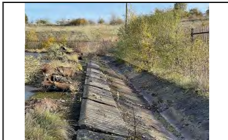
Photo OE/1702/1048/R1/P17 – Concrete lined storm water channel at perimeter of former coal mine site – east side of site – looking north
