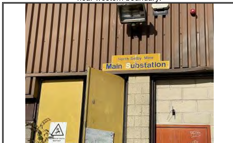
Photo OE/1702/1048/R1/P41 – Existing buildings on the site – main electrical sub-station on the site – near western boundary.
