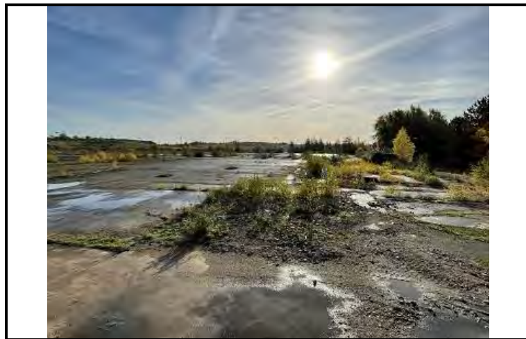
Photo OE/1702/1048/R1/P08 – General view of site and exposed concrete slabs - looking southeast.
