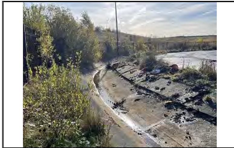
Photo OE/1702/1048/R1/P22 – Concrete lined storm water channel at perimeter of former coal mine site – north side of site – looking east.
