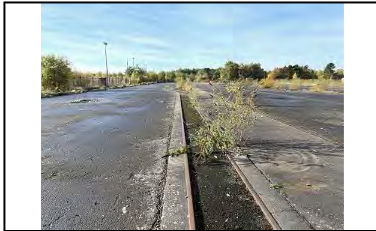
Photo OE/1702/1048/R1/P19 – View of mineral railway line within concrete slabs, near to eastern boundary and landscaping area.
