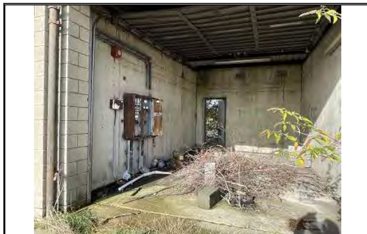
Photo OE/1702/1048/R1/P30 – Inside a building on the western side of the site.
