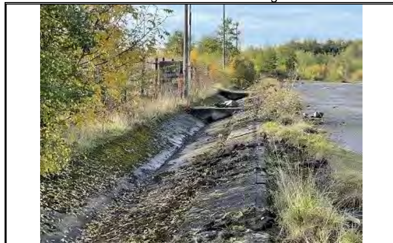
Photo OE/1702/1048/R1/P18 – Concrete lined storm water channel at perimeter of former coal mine site – east side of site – looking south
