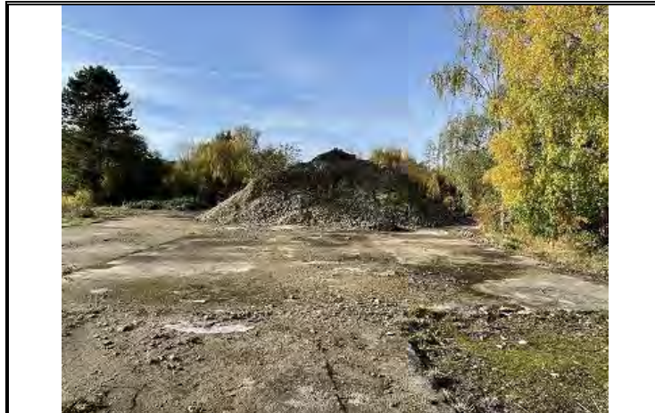
Photo OE/1702/1048/R1/P44 – Existing mound of crushed demolition waste – sampled and tested – see RSK Phase II Report 2021.
