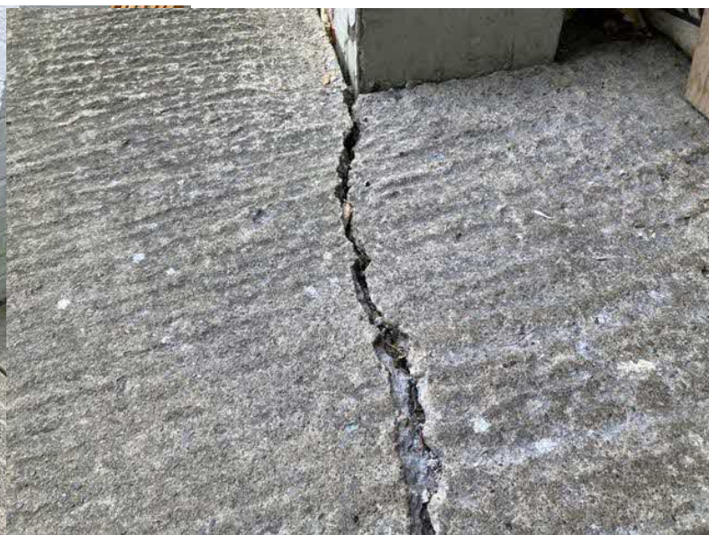
Detritus etc within crack
