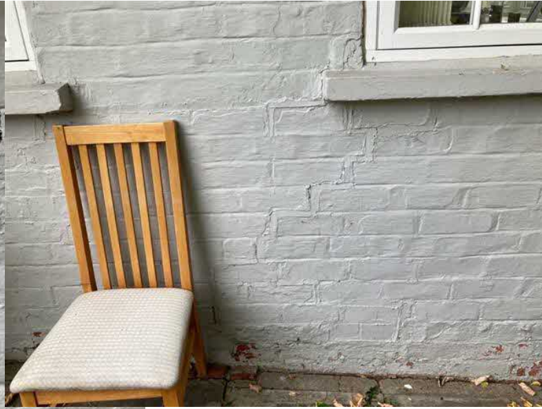
Crack to right side of bay
