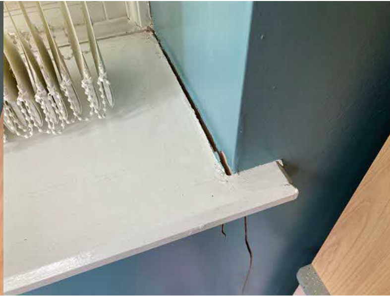
Gaps to sill above lining split.
