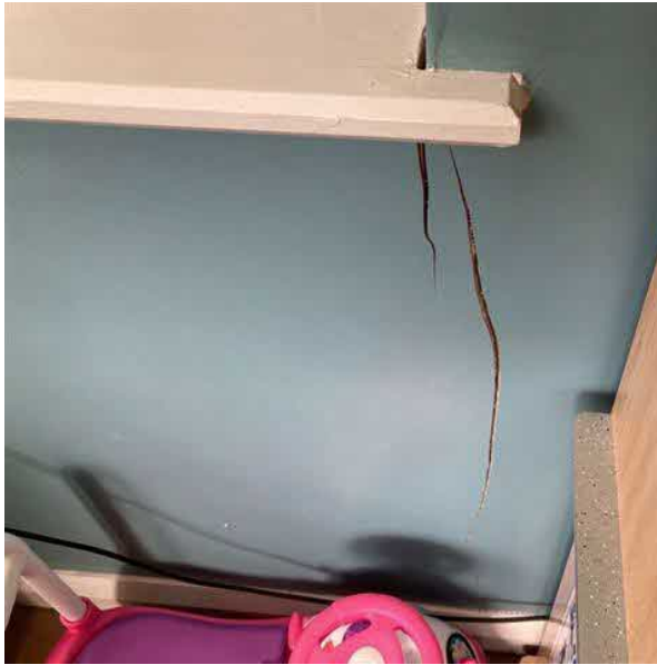
Lounge at join with bay to right elevation. Dry lining split.
