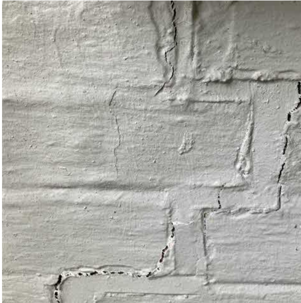
Previous repairs re-opened
