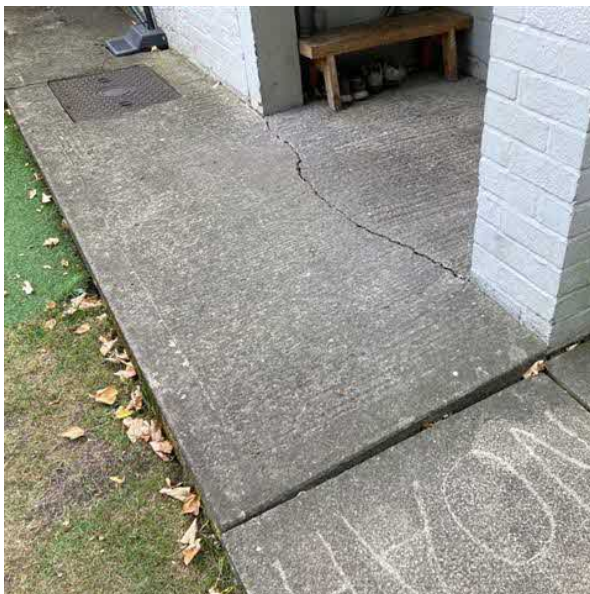
Previously cracked concrete path
