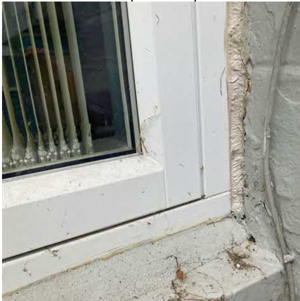
Aged and poorly applied mastic intact to left side of bay
