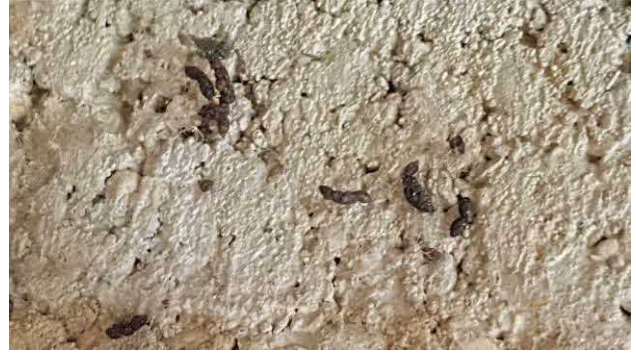
5. Bat droppings in boiler room
