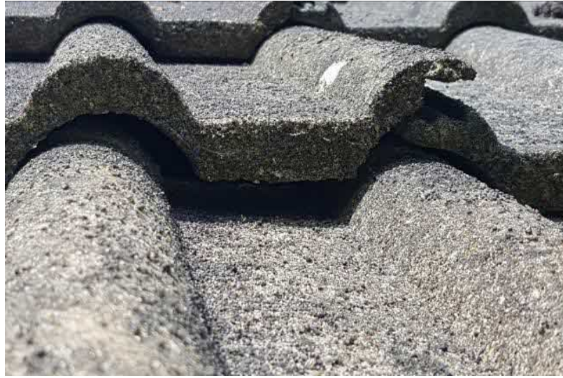
10. Gaps under roof tiles
