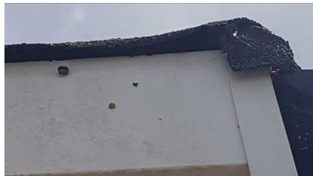
12. Gaps under bituminous felt
