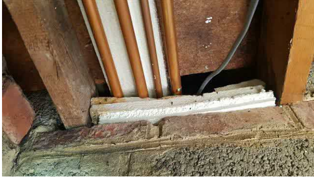
4. Bat droppings in boiler room
