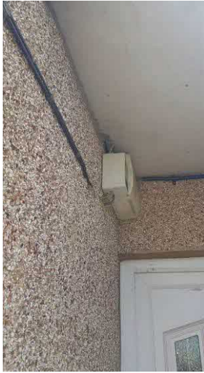
9. Gap into porch roof
