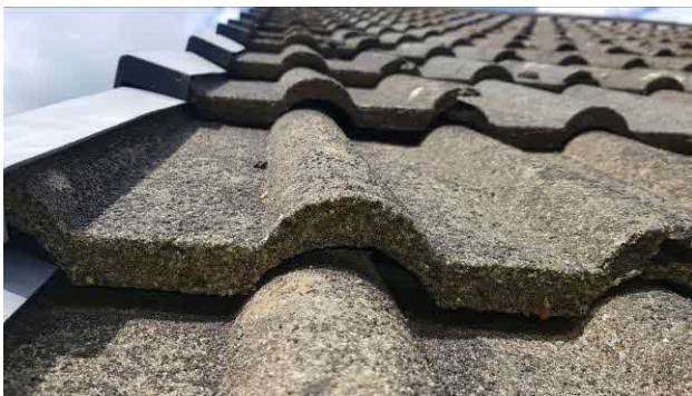
11. Gaps under roof tiles
