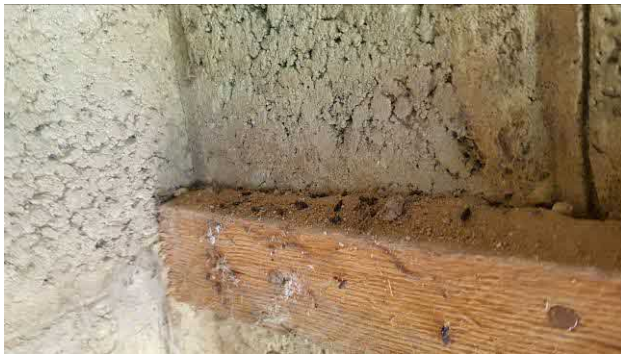
6. Bat droppings in boiler room
