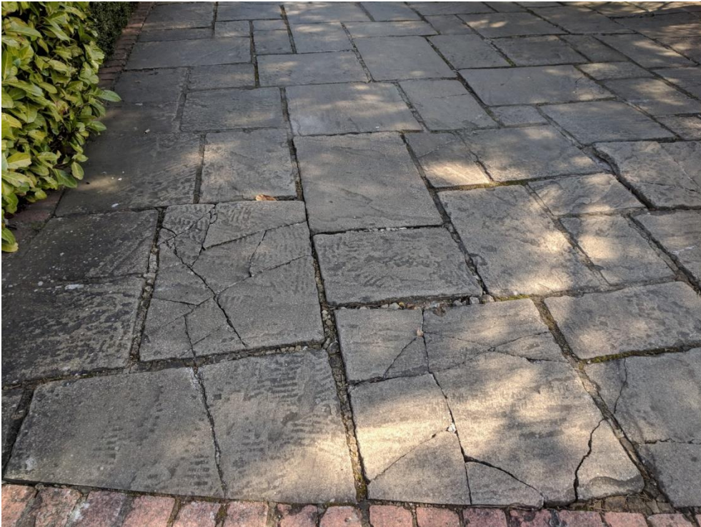
Cracking to paved finishes
