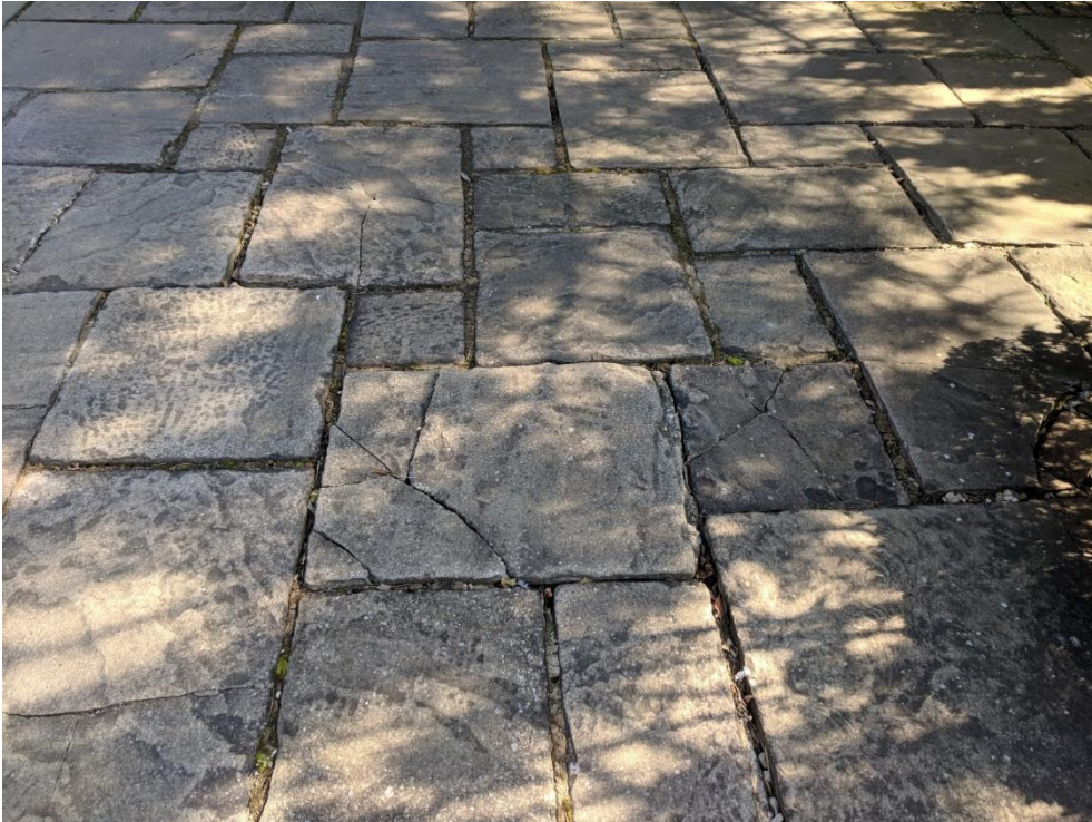
Cracking to paved finishes
