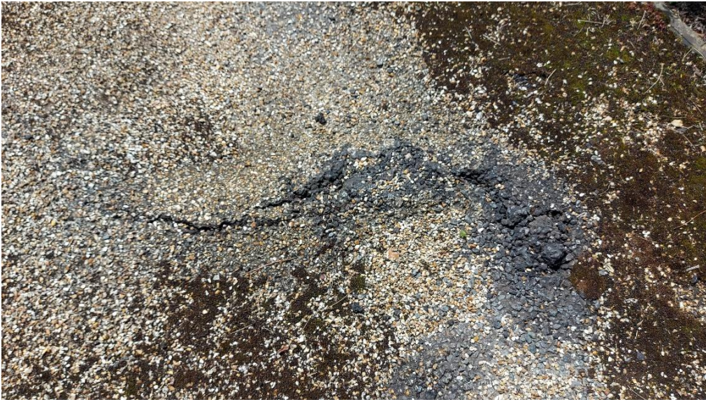
Disturbance to tarmac finishes to driveway to No.2 Percheron Close
