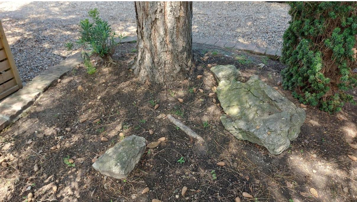
Disturbance to finishes adjacent to base of tree
