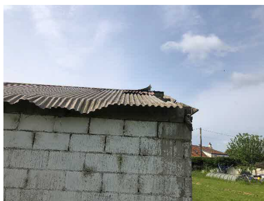
Metal corrugated roofing with multiple holes
