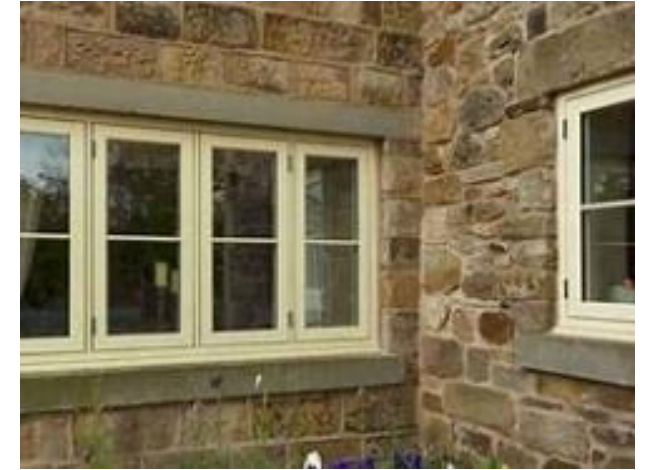
Cotswold biscuit Residence 9 window casements.
