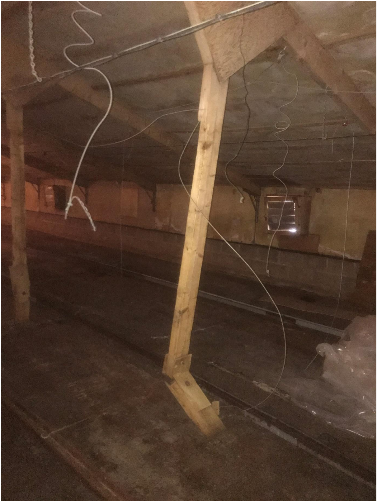
Photograph 7 – Broken Post to Frame '3'
