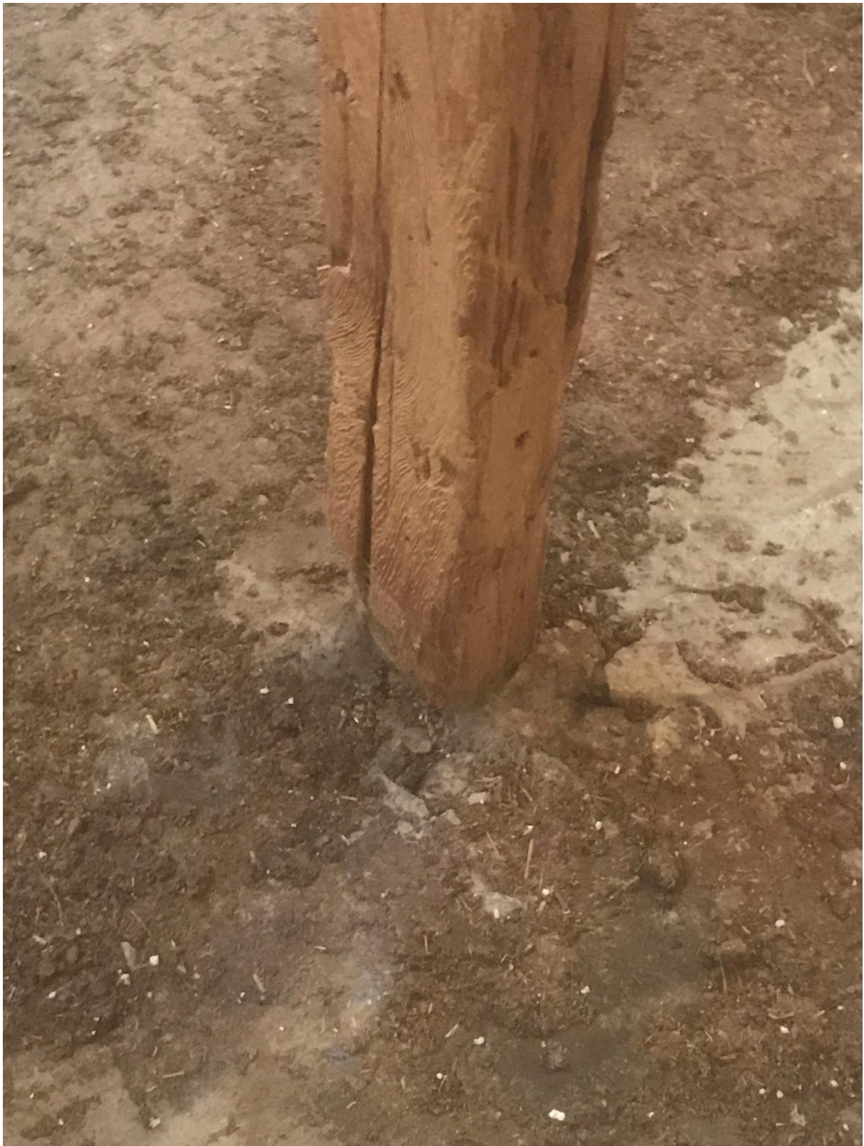
Photograph 10 – Deterioration to Foot of Post
