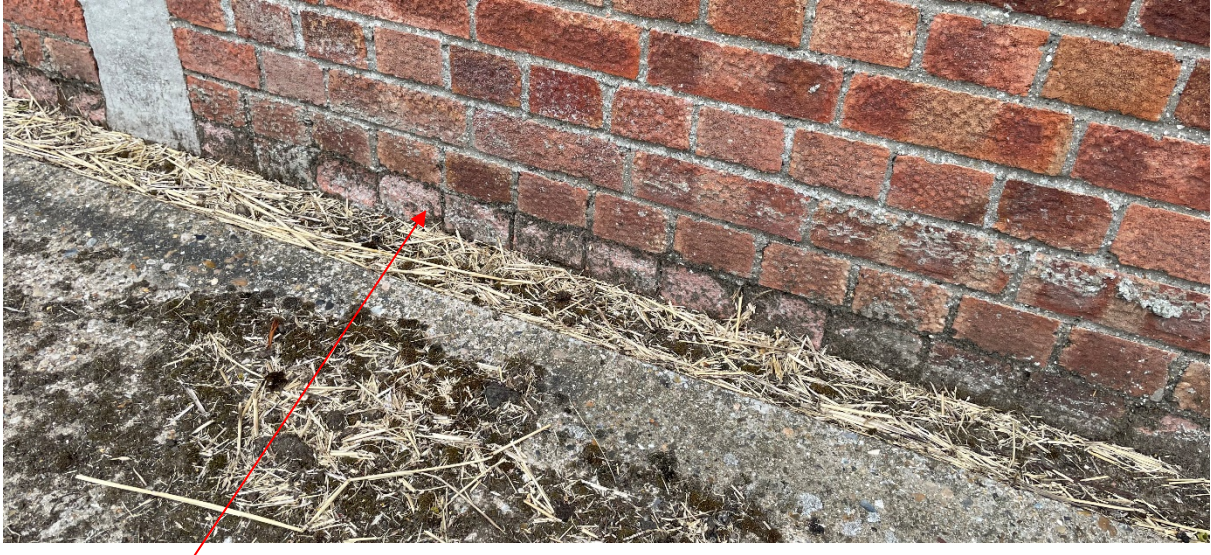
Minor deterioration to bricks at low level
