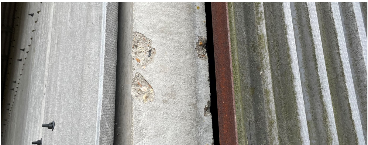
Minor deterioration to face of concrete frame section
