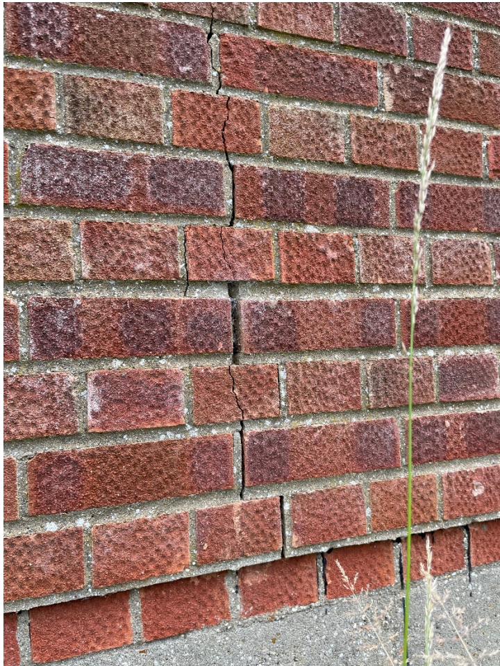
Cracks resulting from impact damage
