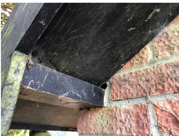
Photo 7: Gnawed hole in south eastern soffit of Building 1
