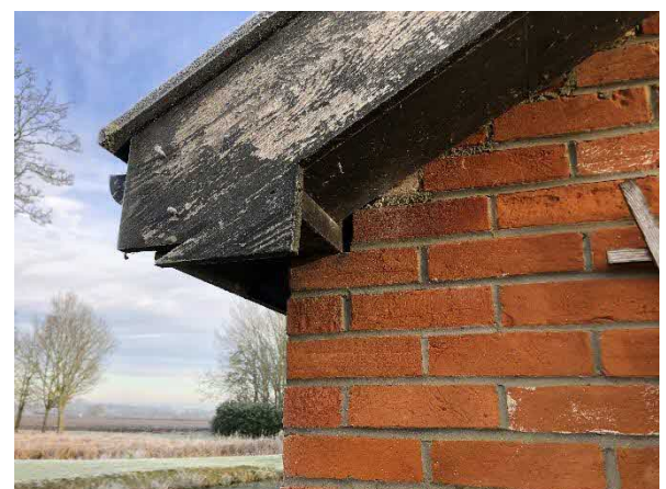
Photo 8: Gap around soffit on north western corner of Building 1
