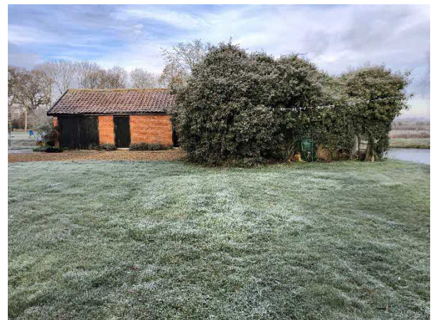
Photo 2: Southern facades of B1 and B2, adjoined by amenity grassland and gravel
