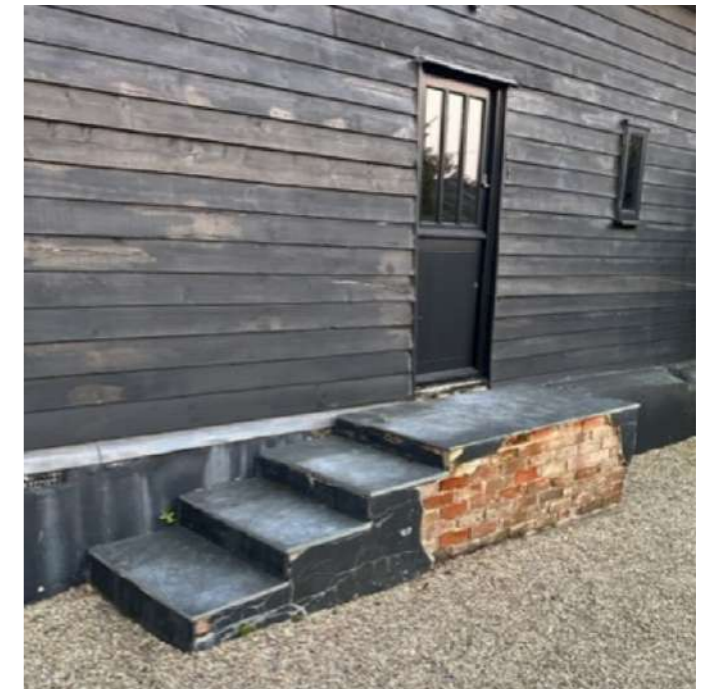
8 - External view of door to be removed. Steps to also be removed and plinth rendered and painted black to match existing.
