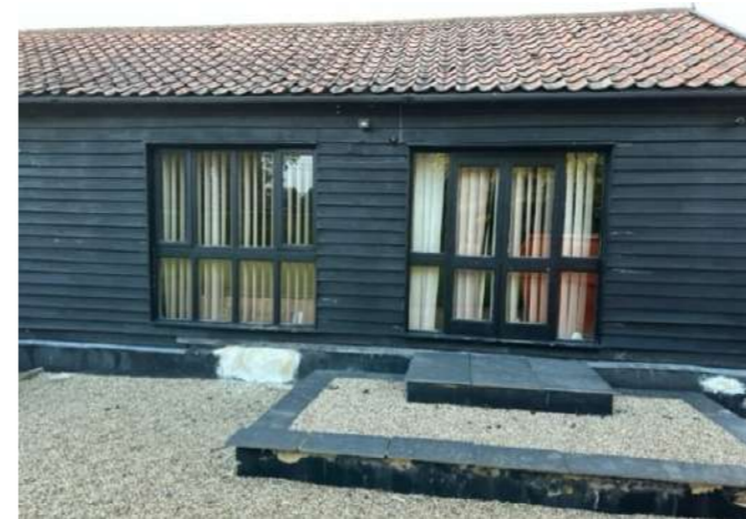
6- Existing full height timber screens to annexe to be replaced.
