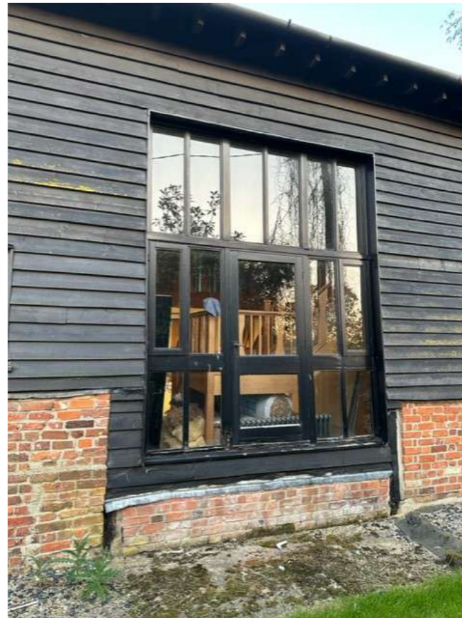
11 - Existing glazed screen within historic barn opening. New bespoke timber glazed screen to be fitted without door. Screen to be divided into 6 panels with mullions as indicated within the upper part of the existing screen.
