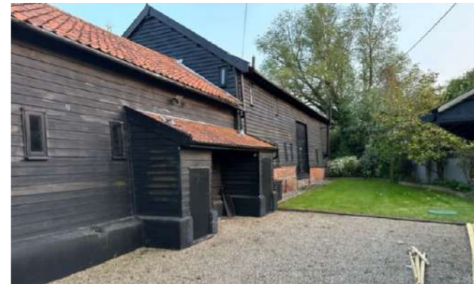
13 - Existing lean-to boiler cupboards to be removed and new entrance porch constructed.
