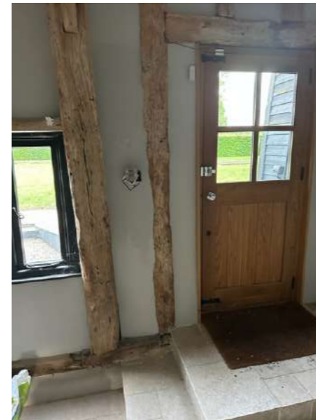
12 - Existing steps over sole plate to be removed. Door and adjacent partitioning to original frame to be removed to form new opening into Garden Room.
