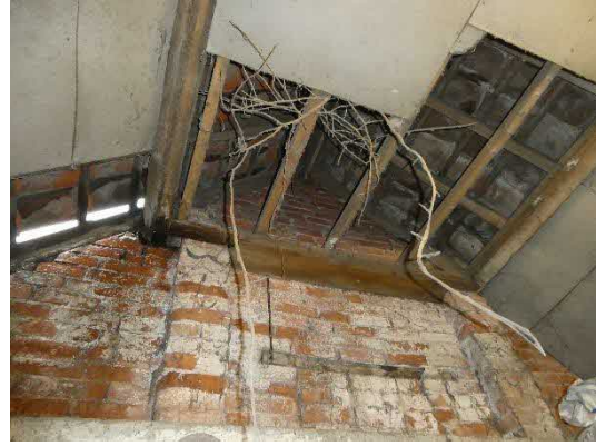
Photograph 12: Outbuilding with hole in the roof covering
