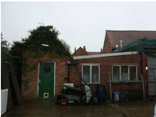
Photograph 9: Exterior view of the link extension and the outbuilding at the west
