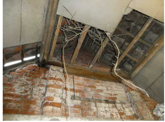
Photograph 12: Outbuilding with hole in the roof covering
