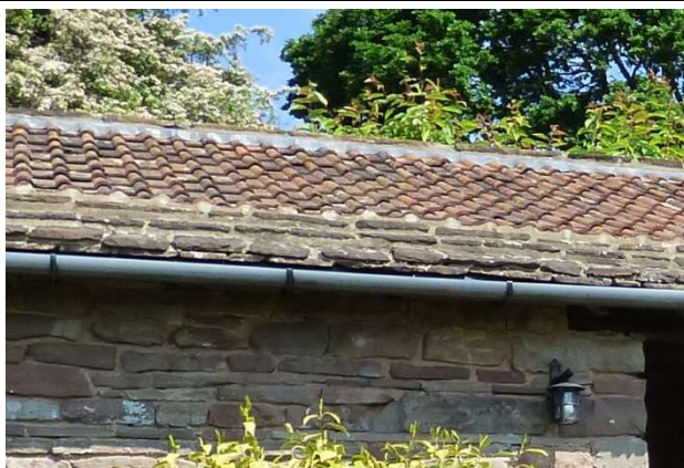
4 – A few gaps under roof tiles were evident but were not common.
