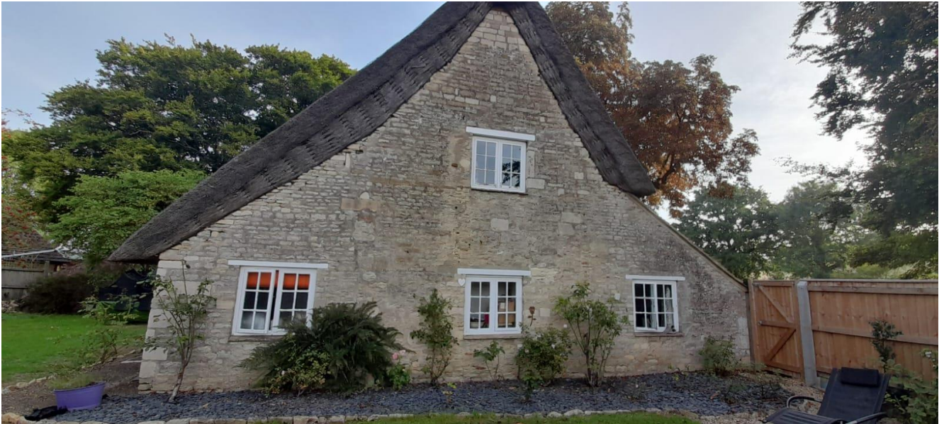
View of the front south west facing front elevation of the cottage prior to replacement windows installation
