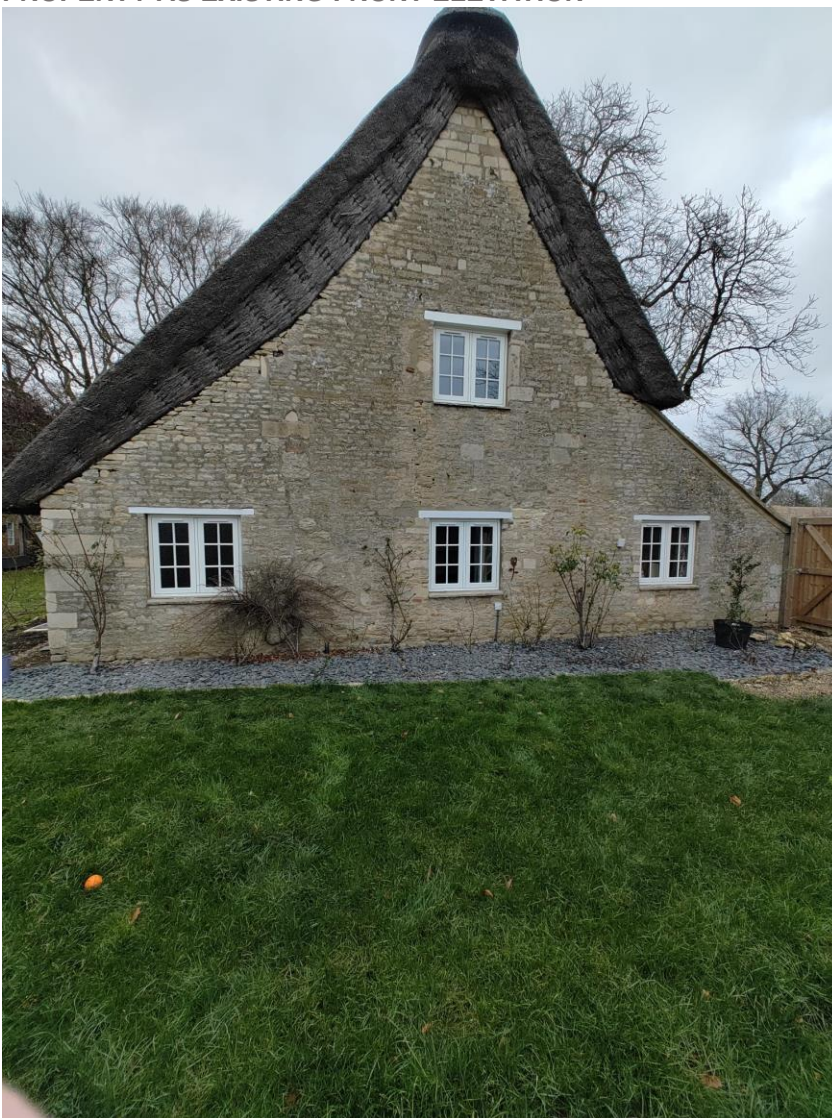
View of the front south west facing front elevation of the cottage as existing
