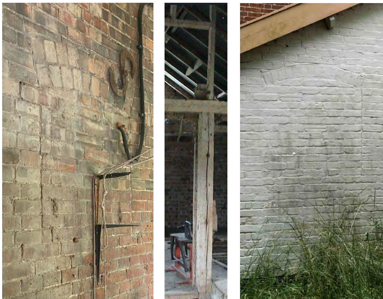
Figure 15. The existing fabric shows marks of the continuous evolution of the buildings on site.
