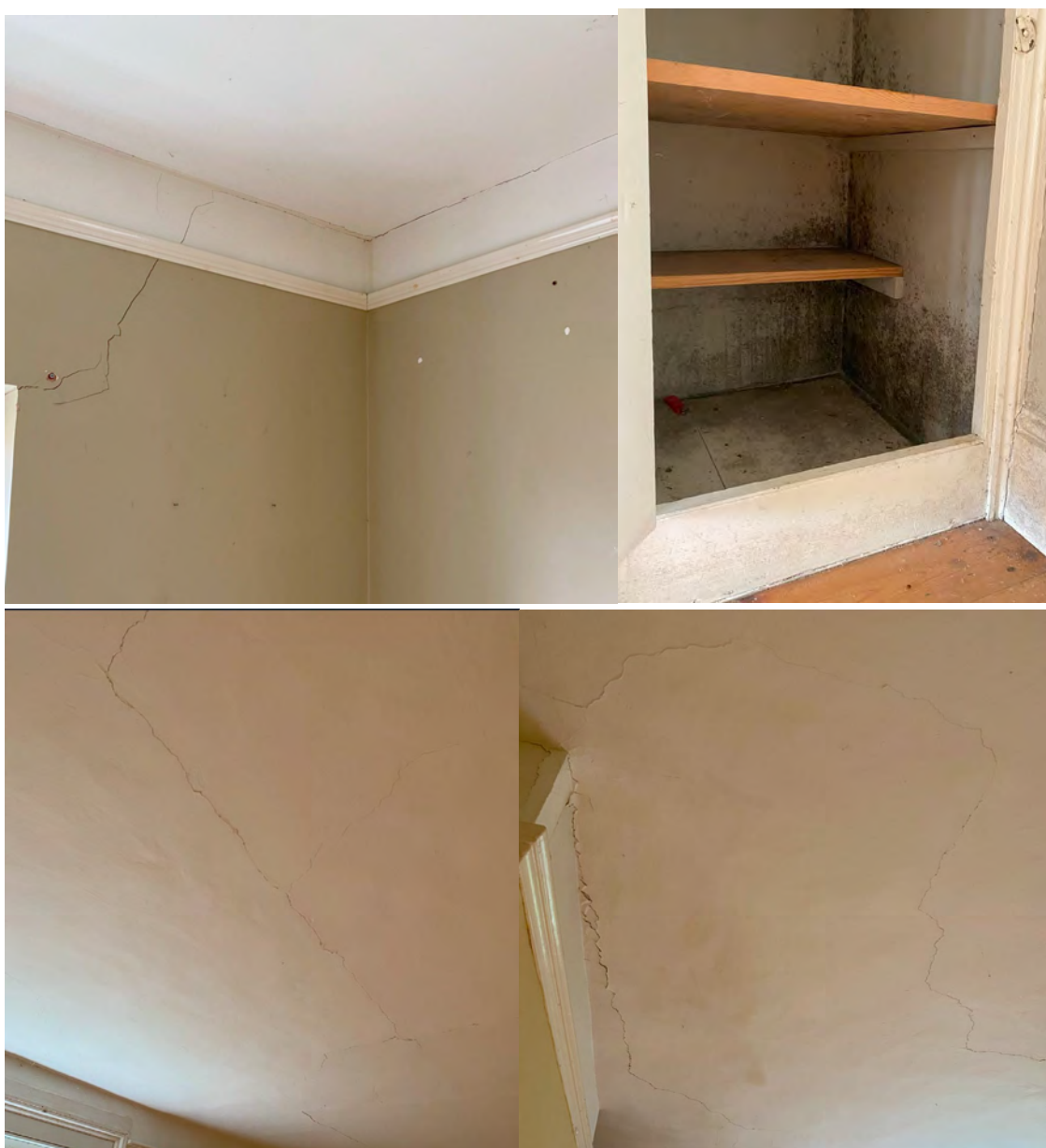
Figure 10. A few examples of cracks found across the Edwardian extension that suffers from subsidence and mold
